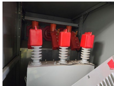
Power Factor Correction Capacitors that were placed into service
