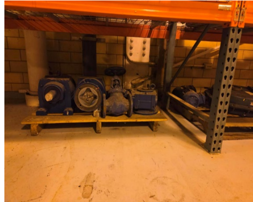
Large machine parts grouped together and stored safely
