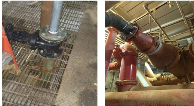
Left: Incinerator No. 7 mist eliminator valve, Right: Incinerator No. 11 SFE strainer backwash elbow
