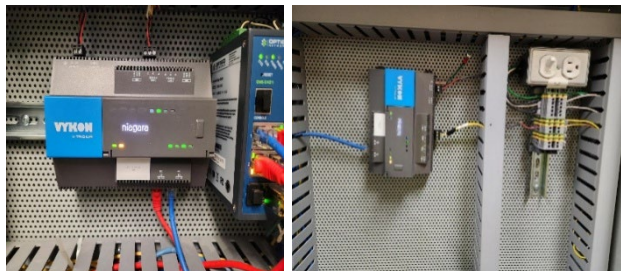
Examples of the new JACE 9000 Controllers installed
