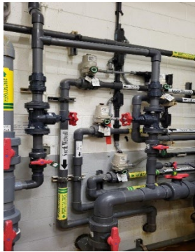
Flushing System integration into the Ferric Chloride System piping
