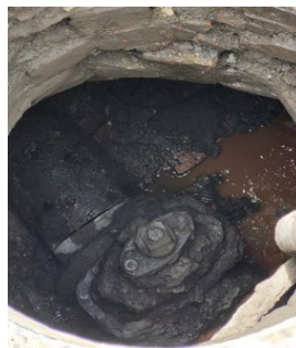
Valve located underground at Stage 3 – Michigan and Rosa
