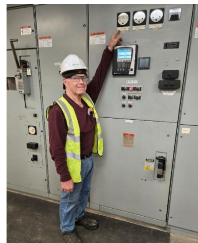
Power Management Electrician George Barnette pointing to the obsolete High Temperature Relay
