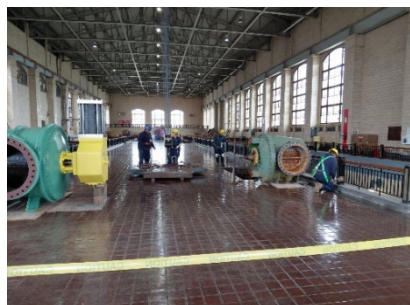
High-Lift Pump No. 22
