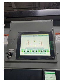
New PLC/HMI installed in EB-26
