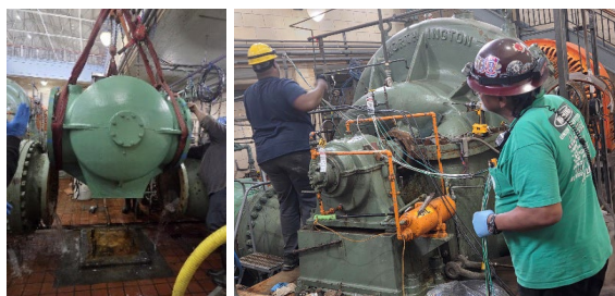
Maintenance Technicians and Electricians
