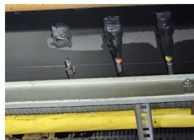
Motor connection damage
