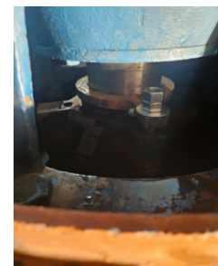
Pump No. 9 at Freud Pump Station
