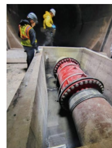
Pinch valve at Oakwood Pump Station
