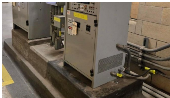
Southwest's battery charging system
