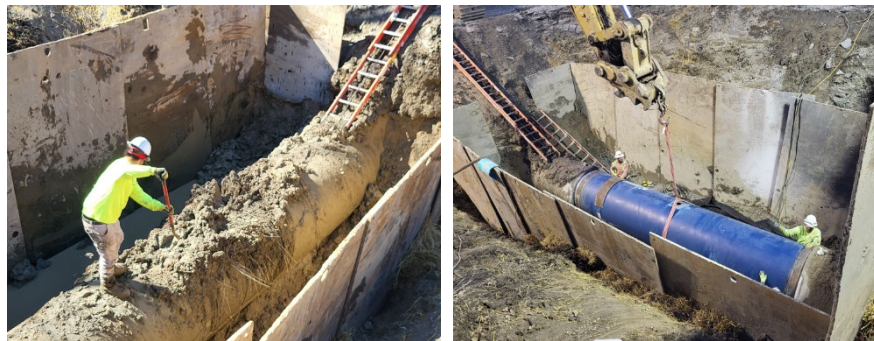
48-inch water main break and repair pipe
