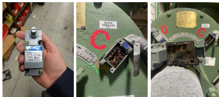
Bad limit switch found on a valve at West Service Center and replaced it with a new one
