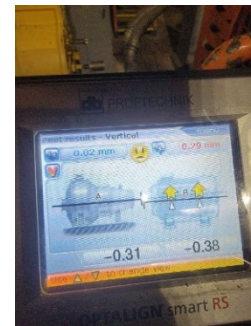
Alignment tool indicating motor adjustment needed
