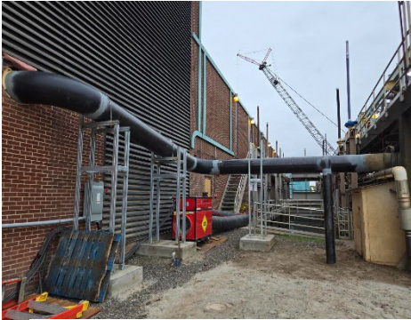
20" Low-pressure Air Bypass
