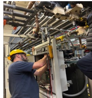
Electrician David Jahn troubleshooting the evaporator
