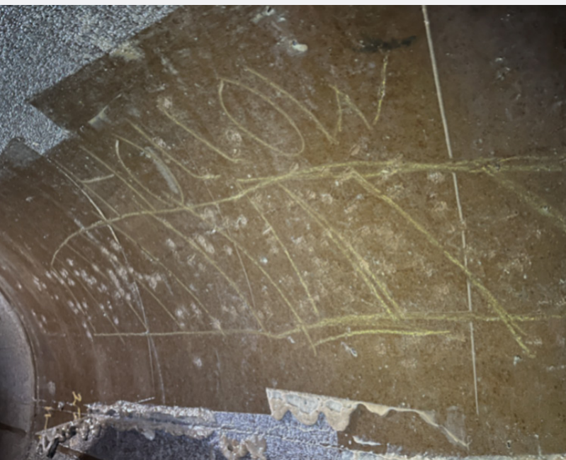
Visual and sounding inspections identified 18 pipes in a state of incipient failure
