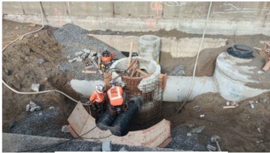
7 th Street Storm Drain
