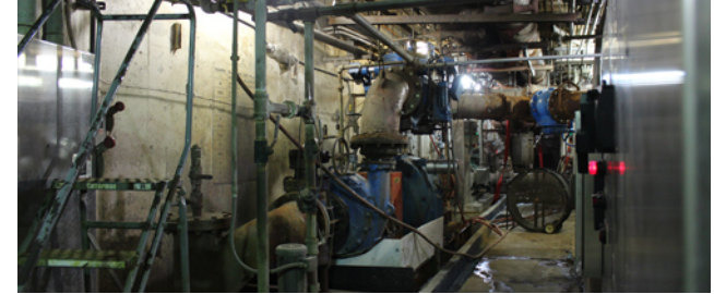
WRRF Improvements to Sludge Feed Pumps at Dewatering Facilities
