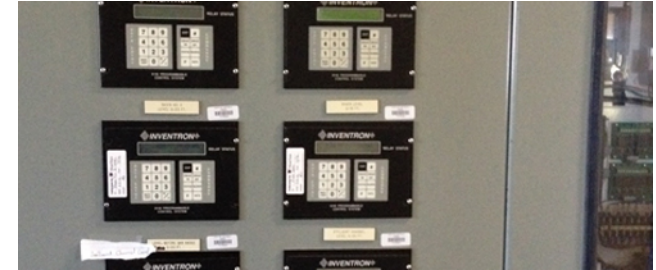
Control System Upgrades at Conner Creek, Oakwood, and Puritan Fenkell CSO Facilities
