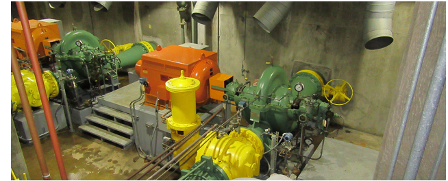
Adams Road Pumping Station
