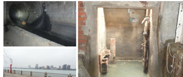
Sewer System Infrastructure Improvements and Pumping Stations
