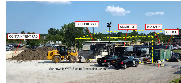
Basins Sludge Processing Facility
