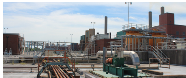
WRRF Aeration Improvements 1 and 2
