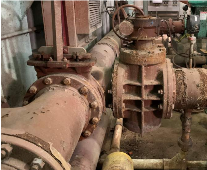
Figure 7-4: Pipe Corrosion and Coating Failures
