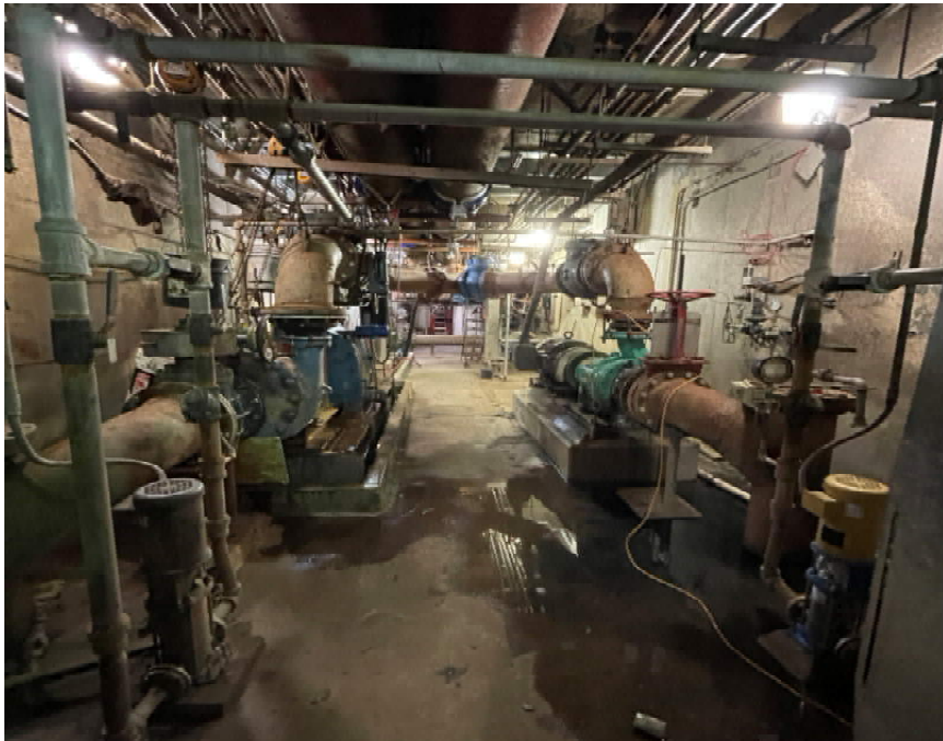
Figure 6-1: SSTs 1-4 Pipe Gallery
