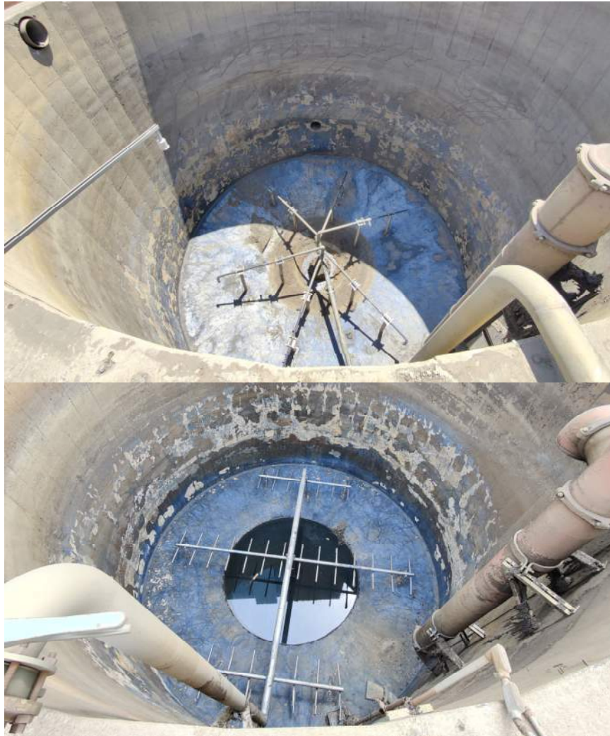
Figure 2-2: Mixing Air Piping and Diffuser Arrangement (SST-1 on top / SST-3 on bottom)
