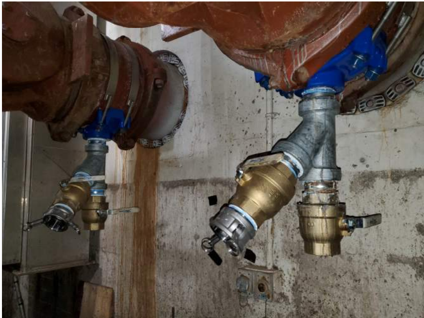
Figure 5-5: SST 5/6 Sludge Inlet Pipe Drainage Ports Downstream of Isolation Valves
