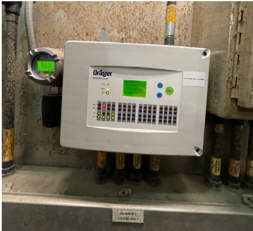
Figure 7-12: SSTs 5/6 Pump Building Hazardous Gas Monitoring System
