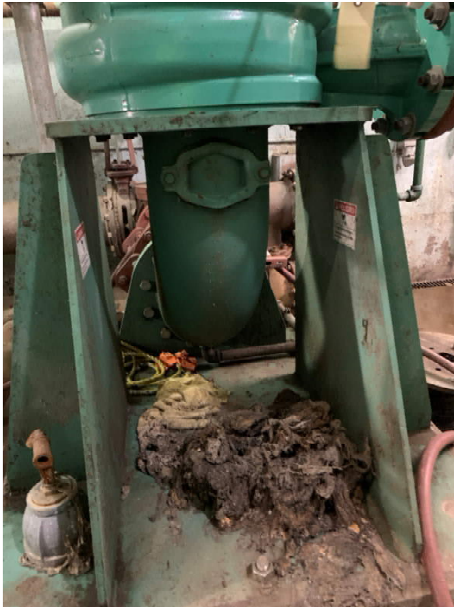
Figure 7-3: SFP-6 Rag Pile on Pump Base Plate
