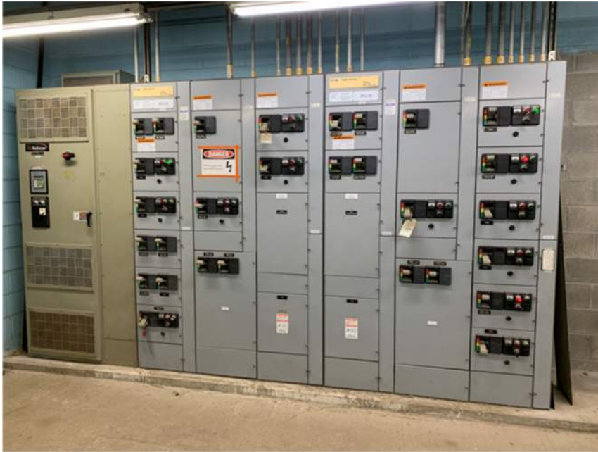
Figure 7-10: MCC-A5 with SFP-5 VFD and MCC-A6
