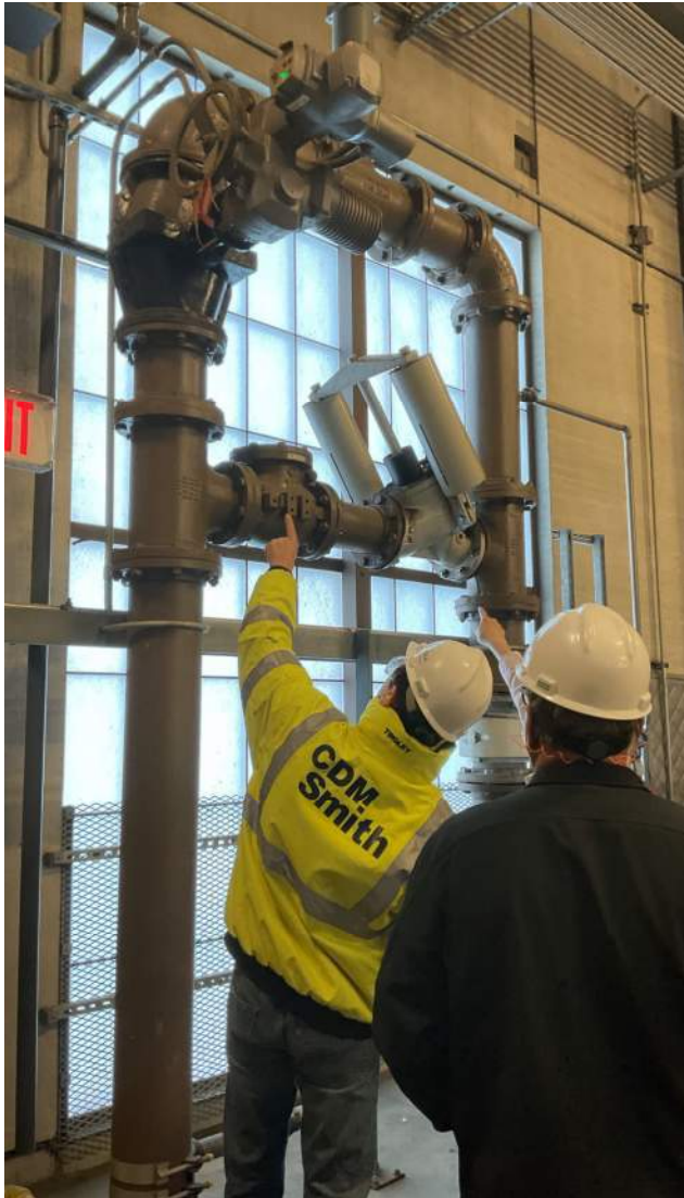
Figure 10-5: Sludge Header Blow-off Manifold
