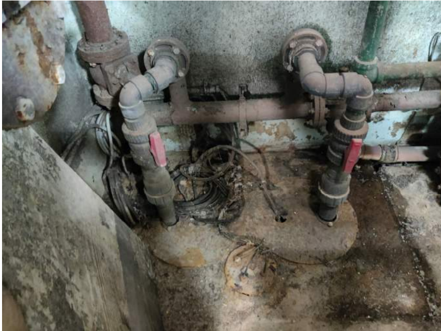
Figure 7-7: SSTs 5/6 Pump Building Sump
