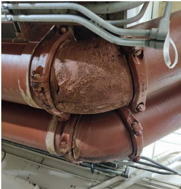
Figure 6-5: Corrosion and Coating Failure on SST Feed Lines
