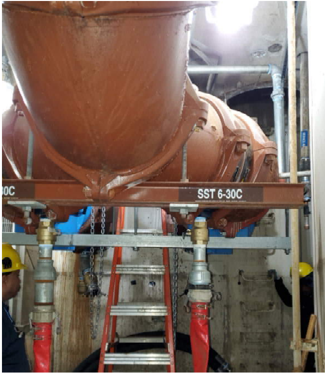
Figure 5-4: SST 5/6 Sludge Inlet Pipe Drainage Ports Upstream of Isolation Valves
