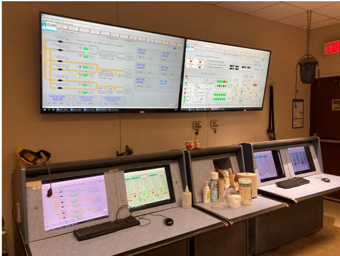
Figure 11-2: S.L. Complex A Ovation Operator Workstations and Large Screen Displays
