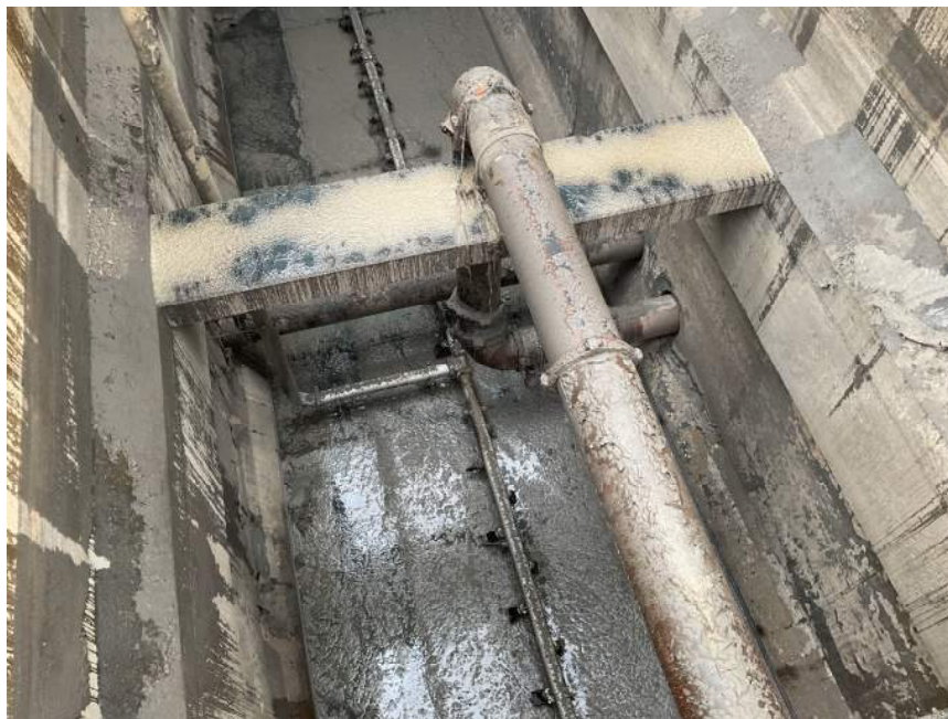
Figure 5-2: SST-6 Mixing Air Piping and Nozzles
