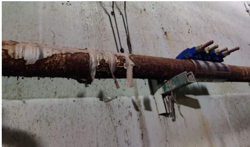
Figure 7-6: Severe Corrosion on Flushing Water Line
