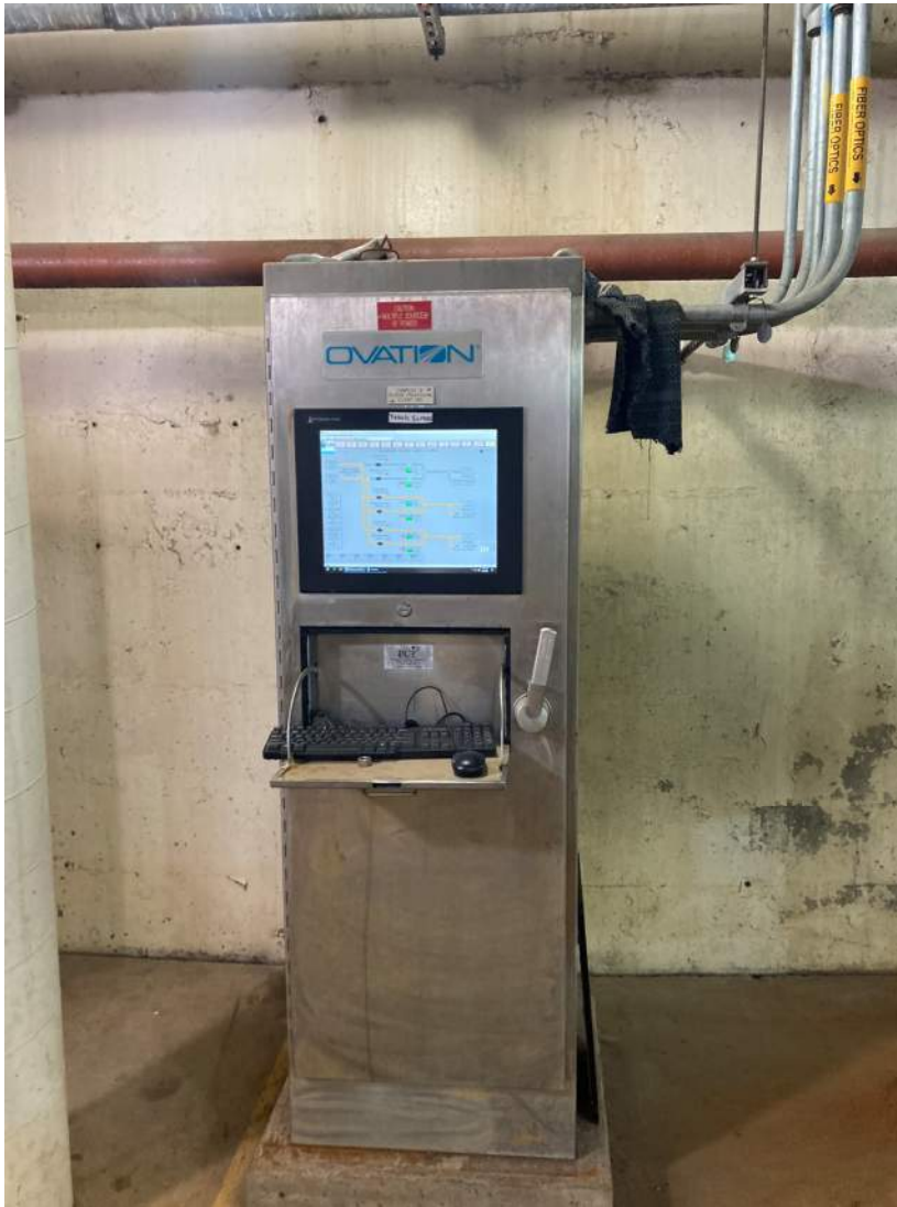
Figure 11-4: Complex A ROS for Ovation HMI Access
