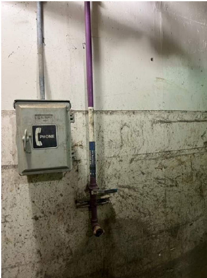
Figure 6-9: 2-inch Compressed Air Line and Quick Connection Below Flood Line
