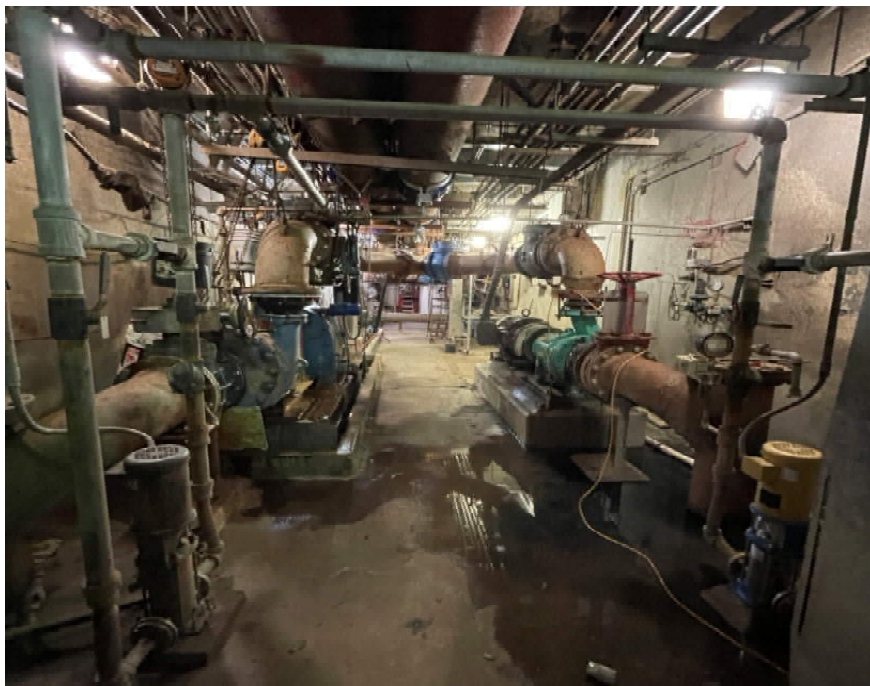
Figure 3-1: SSTs 1-4 Pipe Gallery
