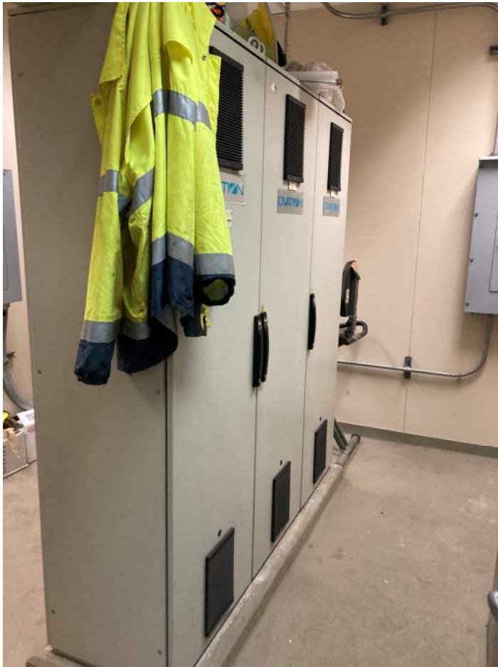
Figure 11-1: Ovation and Network Cabinets S.L. Complex A Equipment Room No. 2
