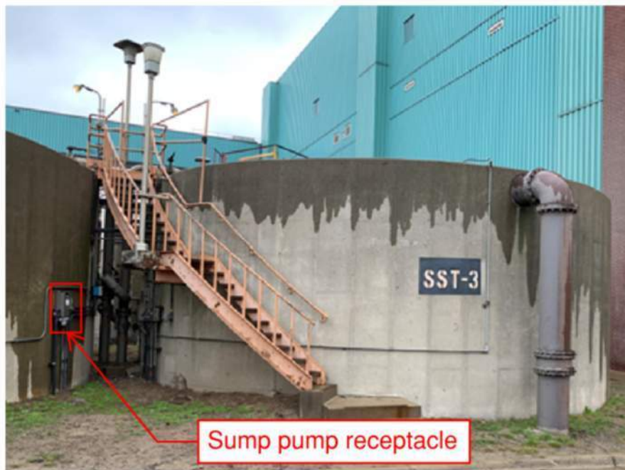
Figure 2-5: Existing SSTs 3/4 Sump Pump Receptacle
