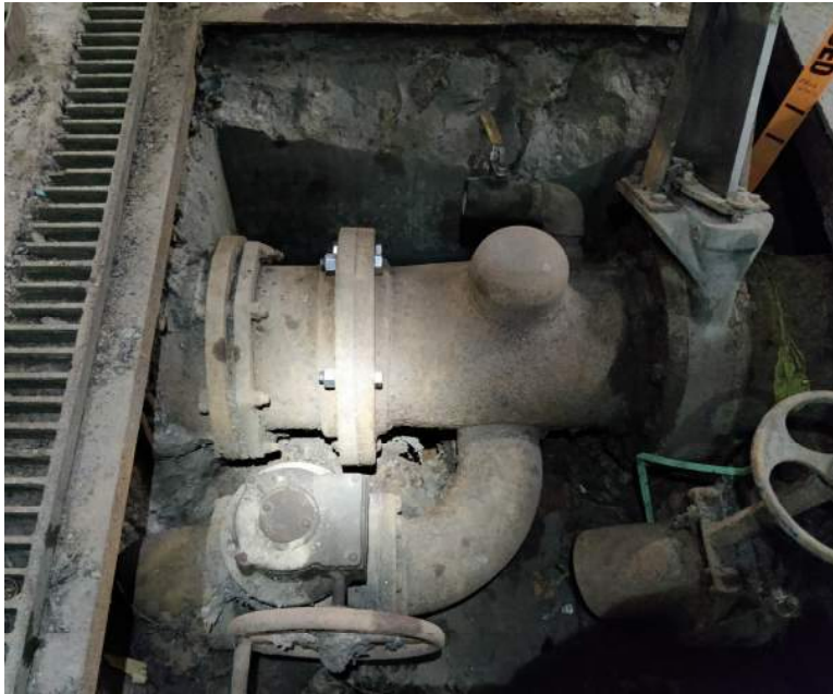
Figure 6-4: Valve Sump on South End of SSTs 1-4 Pipe Gallery
