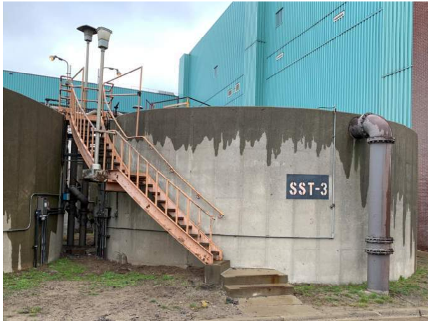
Figure 2-1: Sludge Storage Tank 3 (typical of SSTs 1 to 4)
