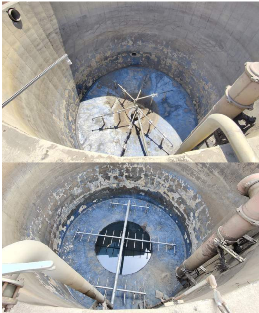
Figure 4-2: Mixing Air Piping and Diffuser Arrangement (SST-1 on top / SST-3 on bottom)
