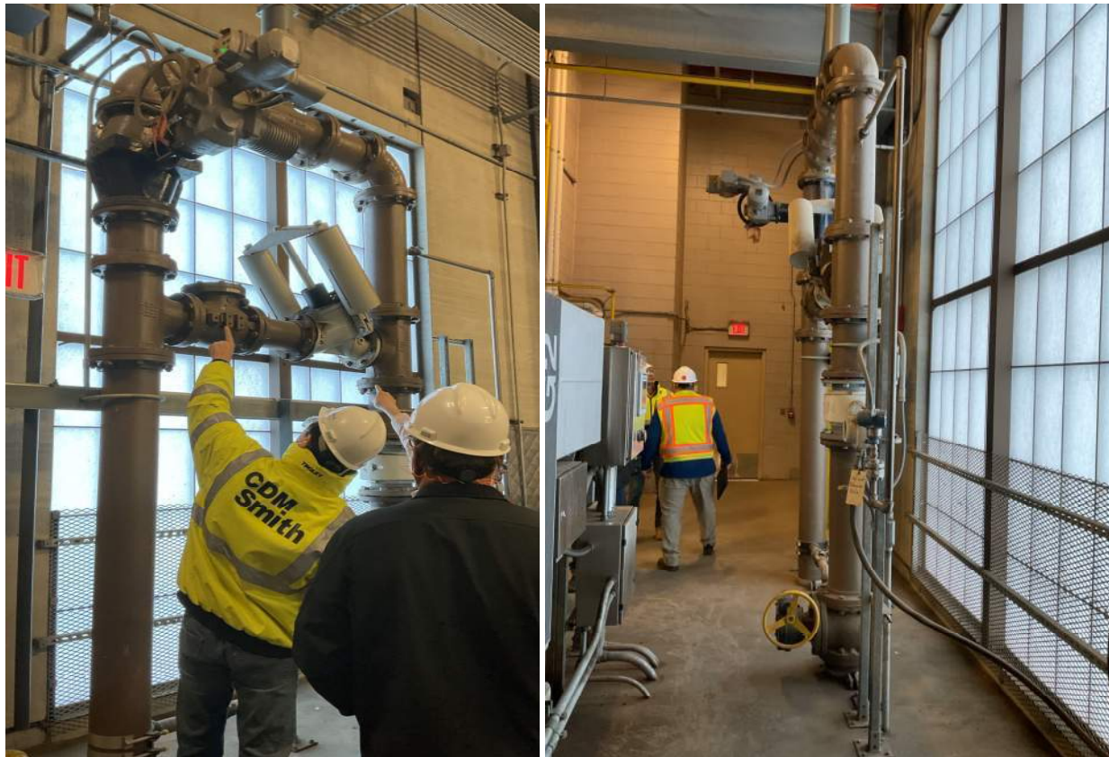
Figure 2-2: BDF Sludge Header Blow-off Manifold (left), Pressure Sensor on Manifold (right)
