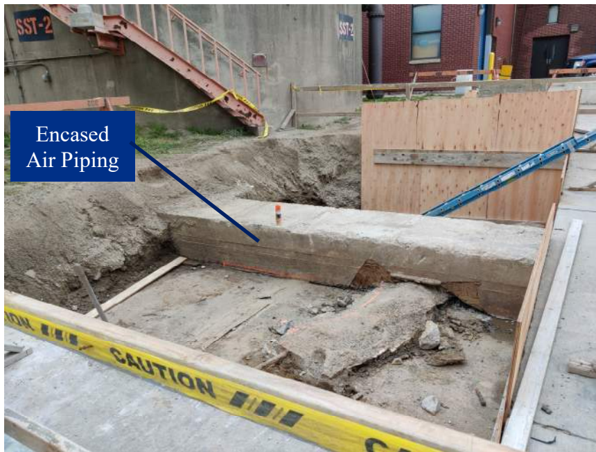
Figure 4-3: Concrete Encased Air Piping above SSTs 1-4 Pipe Gallery (looking west)
