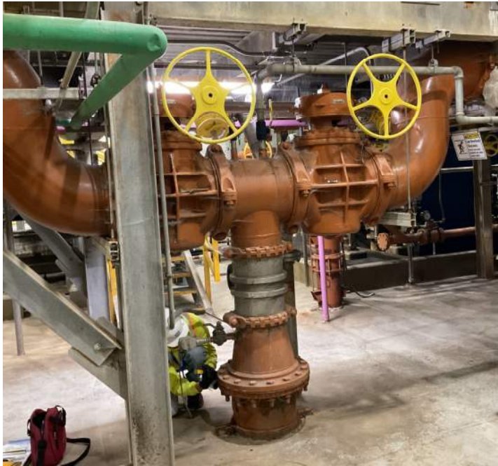
Figure 10-3: Density Meter and 16-inch Header Branches
