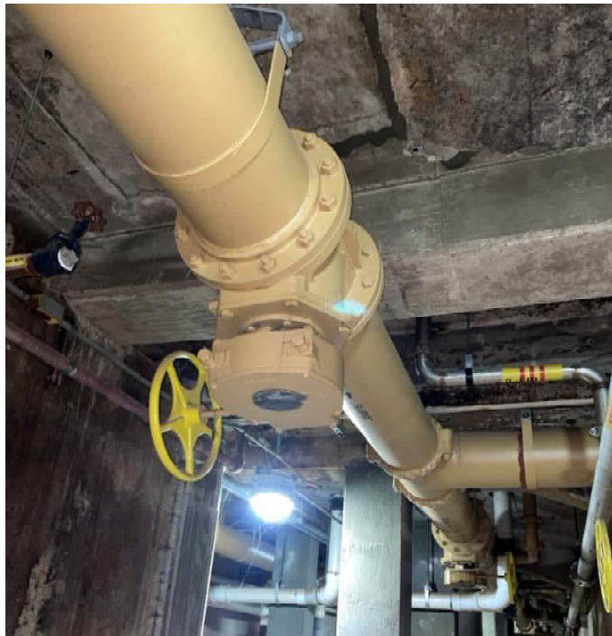
Figure 10-1: Sludge Feed Header in C-I Basement
