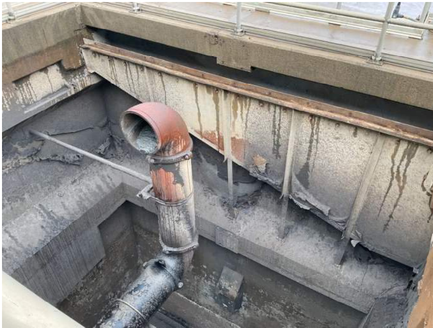
Figure 5-3: SST-6 Sludge Inlet Pipe Discharge and Overflow Weir
