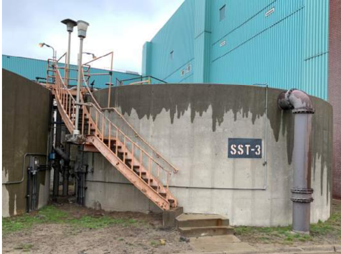
Figure 1.3: Sludge Storage Tank 3 (typical of SSTs 1-4)
