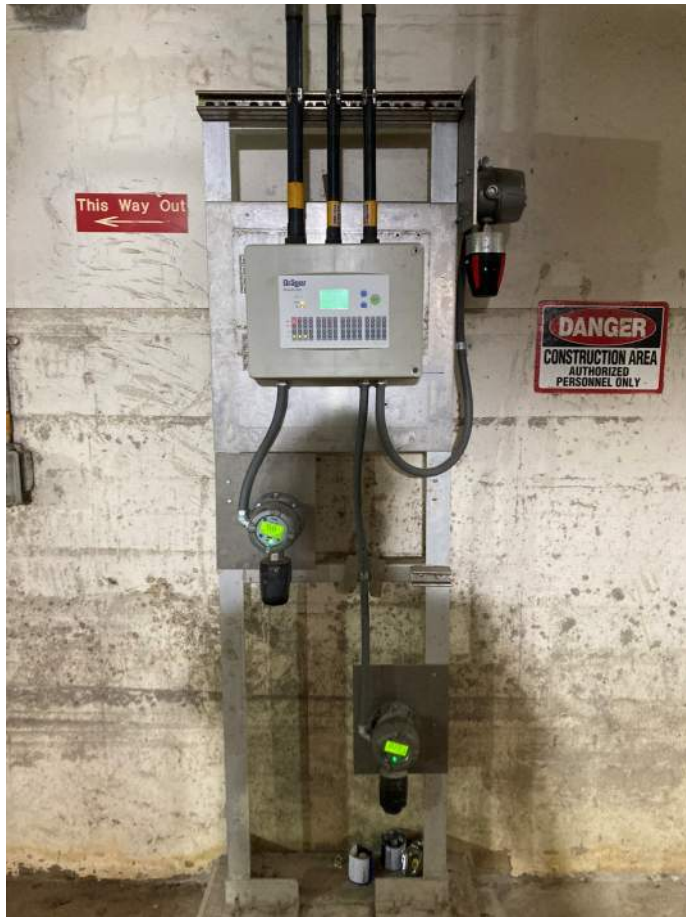
Figure 6-12: Hazardous Gas Monitoring System
