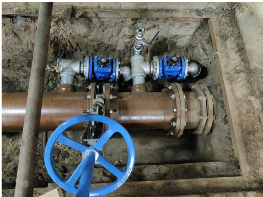
Figure 3-3: Valve Pit on South End of SSTs 1 to 4 Pipe Gallery
