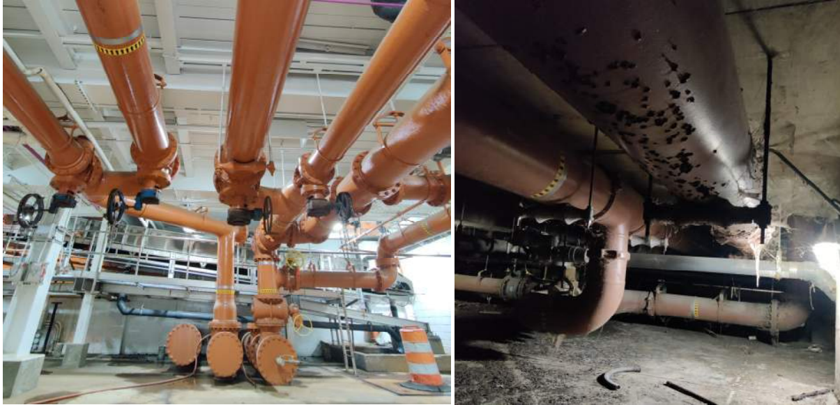
Figure 10-2: Sludge Feed Header to C-II- Entering Basement (left), Through Crawl Space (right)
