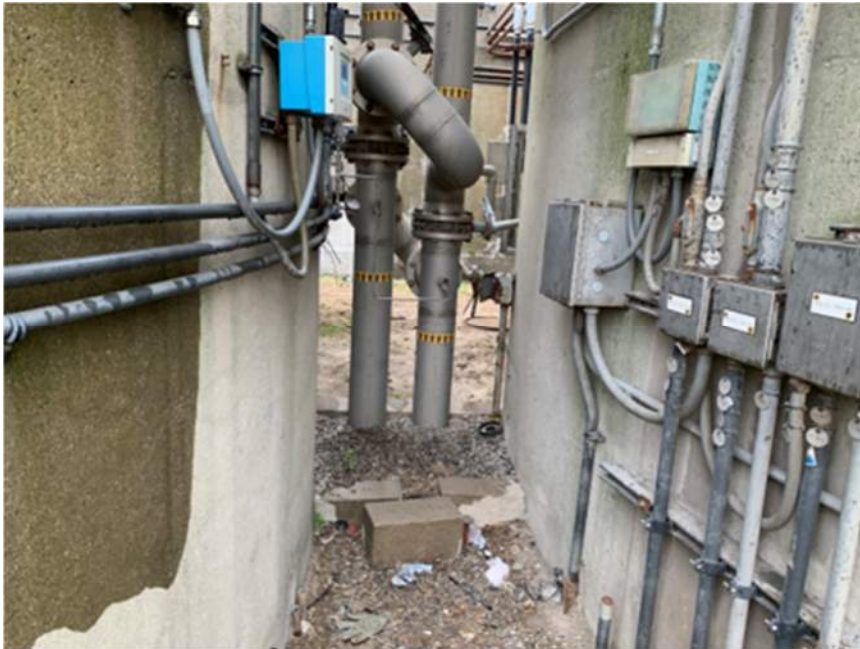
Figure 4-5: Corroded Conduits and Enclosures
