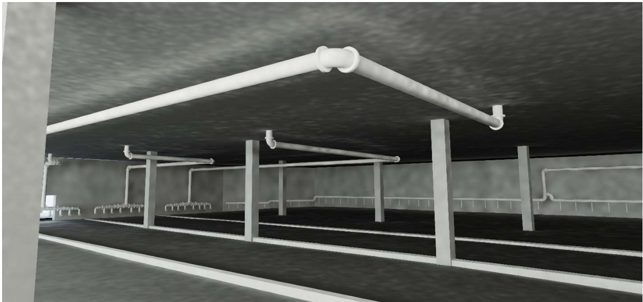
Figure 4-5. Modified Flushing Header Piping along Steeper Sloped Perimeter Areas
