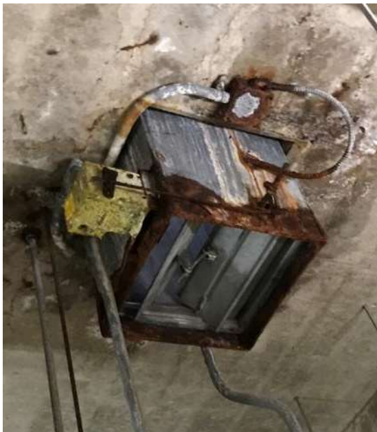
Figure 9-3. Corrosion on EF-7 Ductwork
