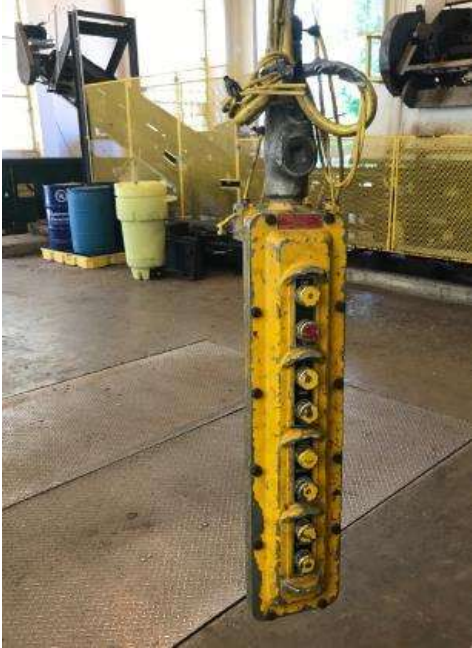
Figure 9-1. Existing Pendant for Overhead Crane at Hubbell-Southfield CSO Facility
