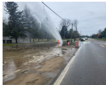
Shelby Township 12-inch water main break on November 16
