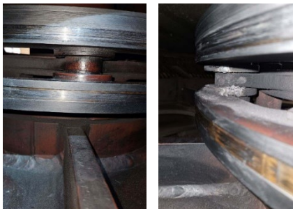
The grounded insulating ring in Main Lift Pump 6 motor and an example of an ungrounded insulating ring shown in the left and right photos above
