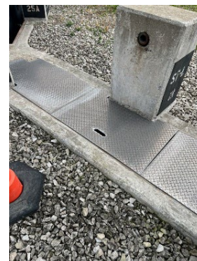
A section of removable floorplates replaced by the Central Maintenance Team to mitigate a fall hazard into a stop log channel
