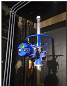
Actuator for one of three gates shown in the photo above
