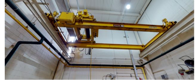
Oakwood HVAC Project
