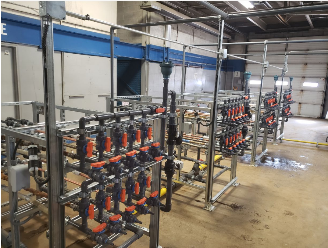
Figure 2-1: Example Pipe Rig Study Setup at One Study Location (from left: Rig D, Rig C, Rig B, Rig A)
