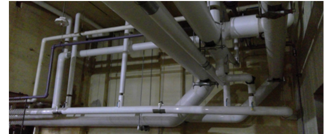
Condensate Return, and Compressed Air Piping
