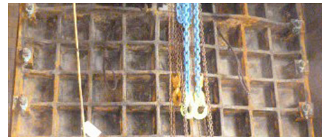
Sedimentation Basin Sluice Gates
