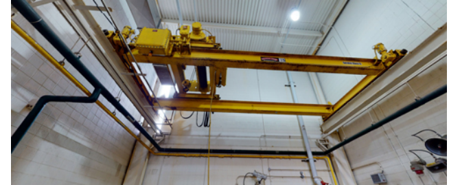
Oakwood HVAC Project
