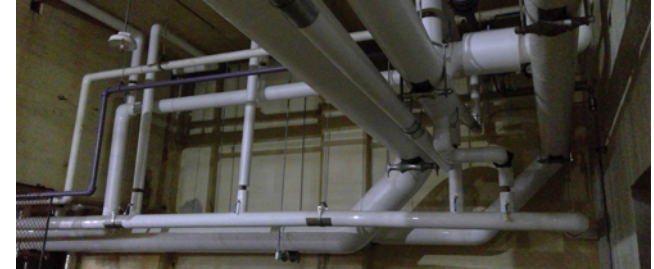
Condensate Return, and Compressed Air Piping
