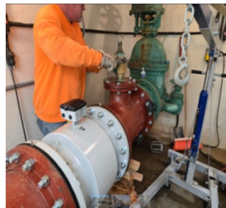
Meter Pit SE-09 14 Mile Road and Lasher
