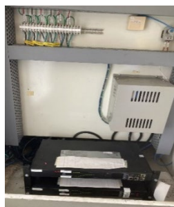
New power transfer switches at WRRF De-Chlorination
