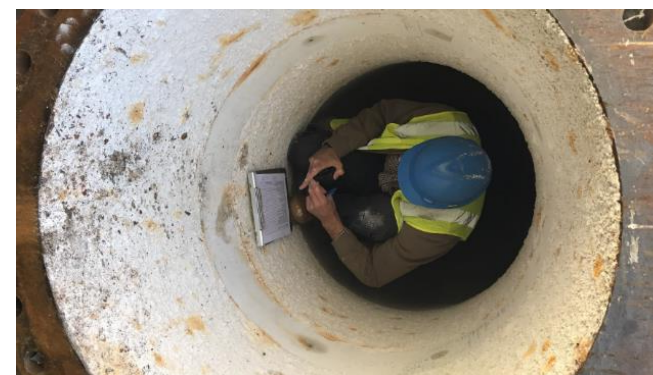
Metering Improvements at Northeast Water Plant
