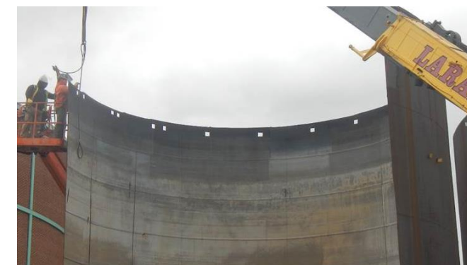
Rehabilitation of Various Sampling Sites and PS#2 Ferric Chloride System at WRRF
