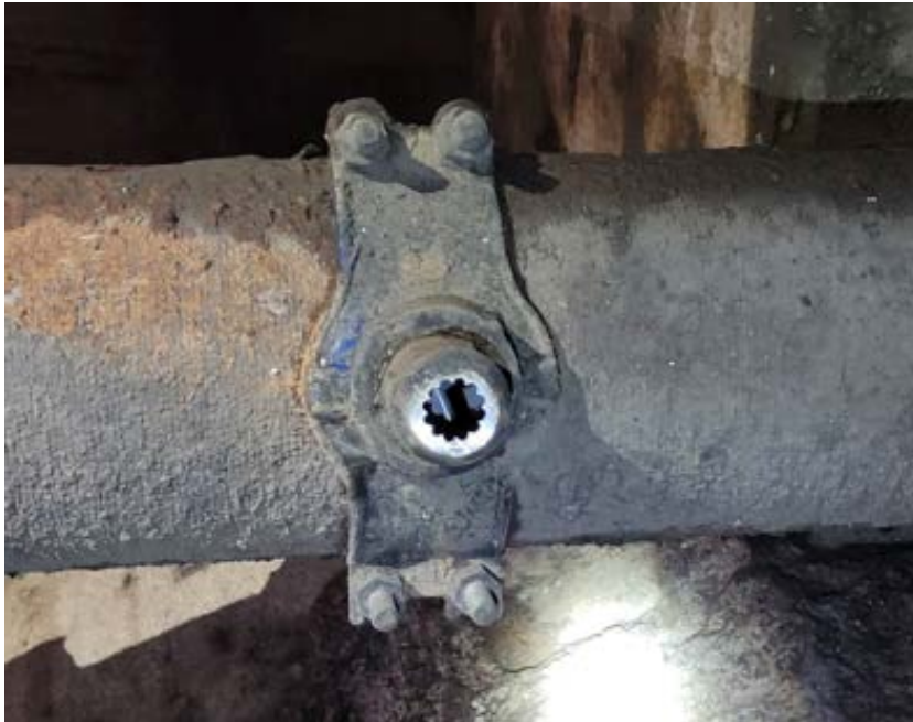
Figure 2-7 Existing Flushing System Nozzle (Oakwood Storm Wet Wells)
