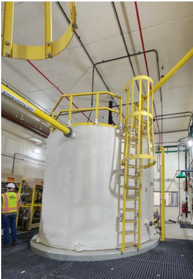
Figure 4-5 Existing Sodium Hypochlorite Storage Tank at Oakwood
