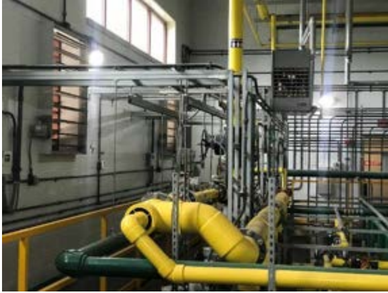
Figure 6-3. Chemical Room Unit Heater Located in Inaccessible Area
