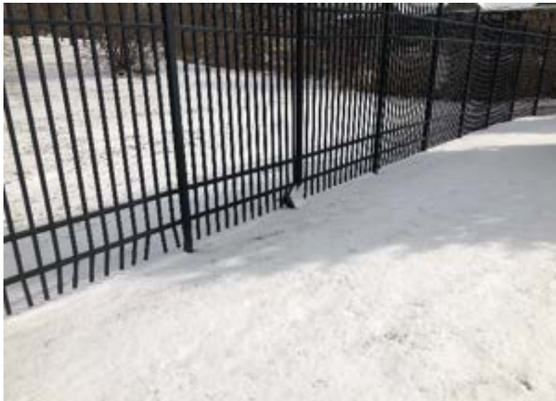
Figure 6-5. Example of Damaged Fencing at Baby Creek CSO Facility
