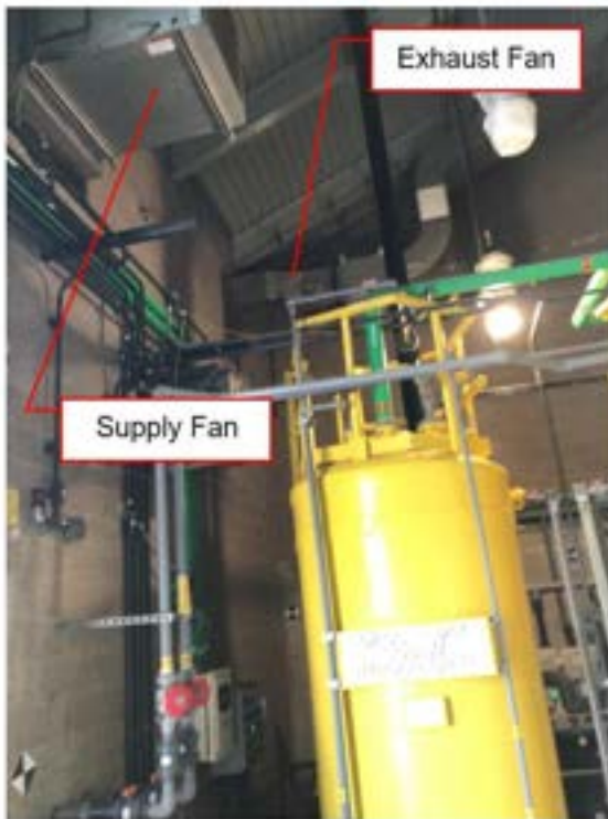
Figure 7-8. Chemical Room Supply and Exhaust Fans Located in Inaccessible Area
