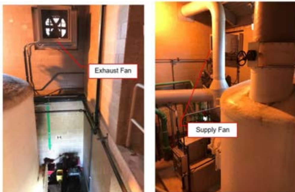
Figure 7-9. Odor Control Room Exhaust (left) and Supply (right) Fan Poorly Accessible
