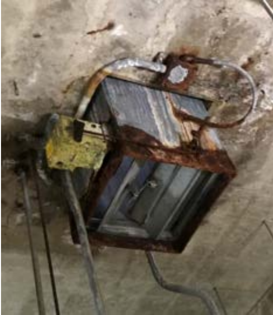
Figure 9-3. Corrosion on EF-7 Ductwork
