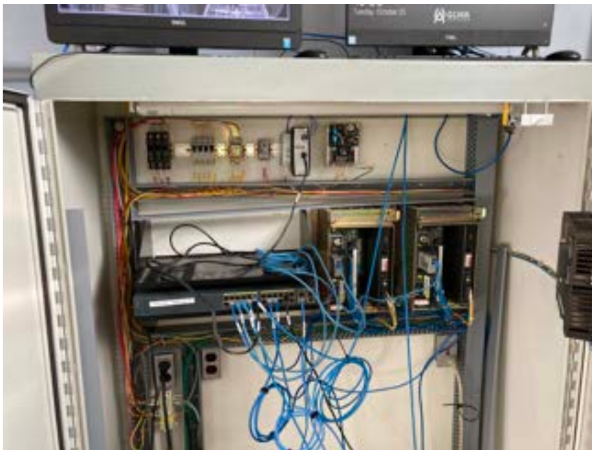
Figure2-7 Existing Allen-Bradley PLC Processor Racks in Office
