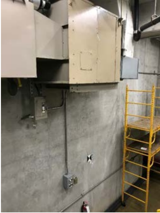
Figure 13-2. HVU-3 Located in Inaccessible Area Difficult to Access Location
