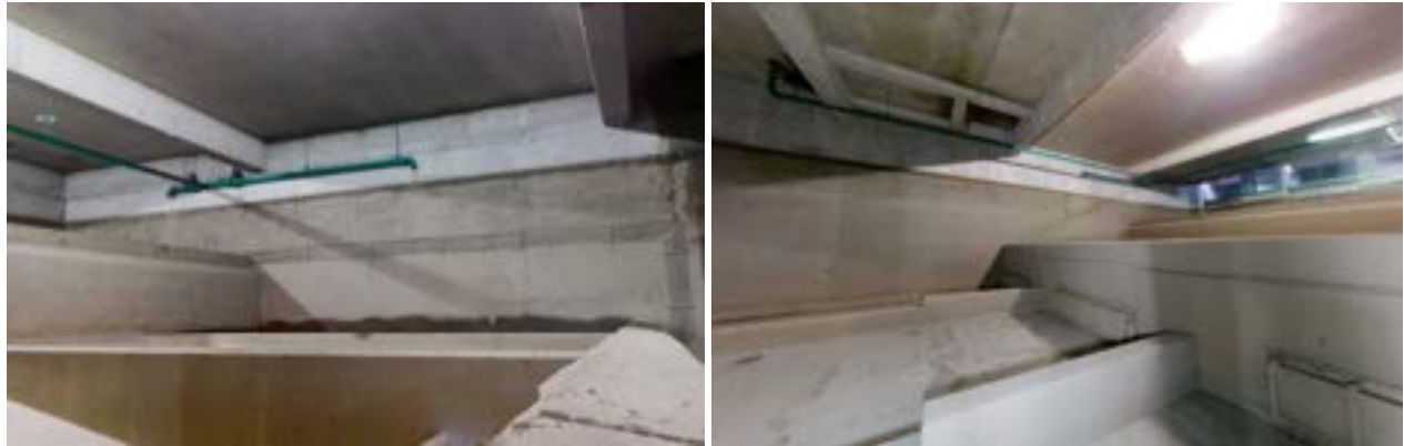
Figure 2-4 Secondary Water Fill Valves for the Flushing Reservoirs (Both) and the Influent Channels (Left)
