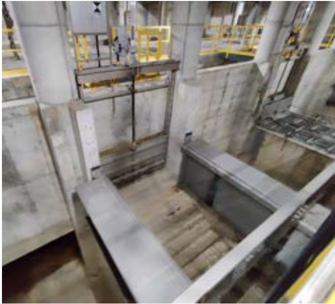
Figure 2-6 Screening Channel Gates for ROMAG (left) and COPA® (right)
