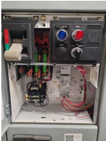
Figure 2-1 Existing soft starter configuration inside MCC bucket
