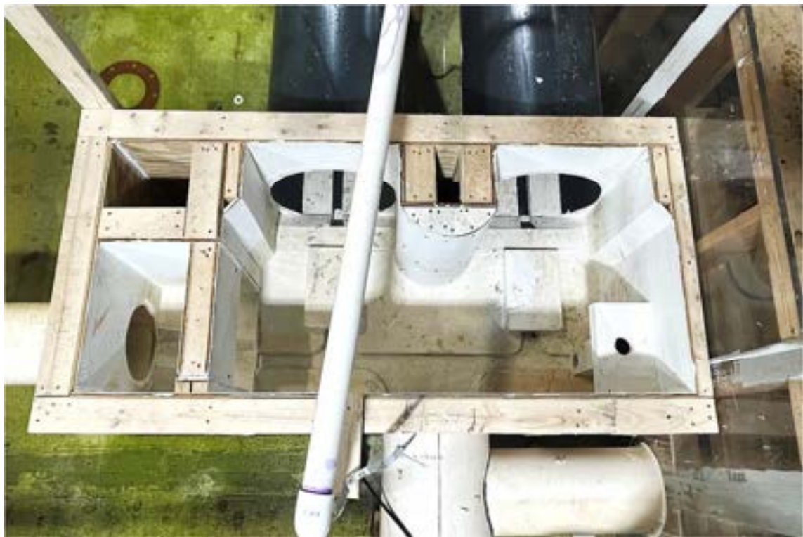
Photo 3-2 Junction / Splitter Box
