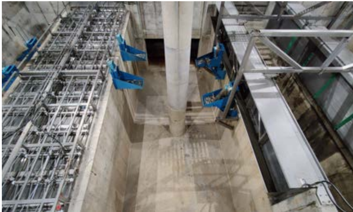
Figure 2-4 Horizontal COPA® (left) and Vertical ROMAG (right) Screens
