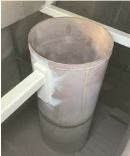
Figure 5-1 Existing Storm Pump Vertical Discharge Piping in Screen Facility
