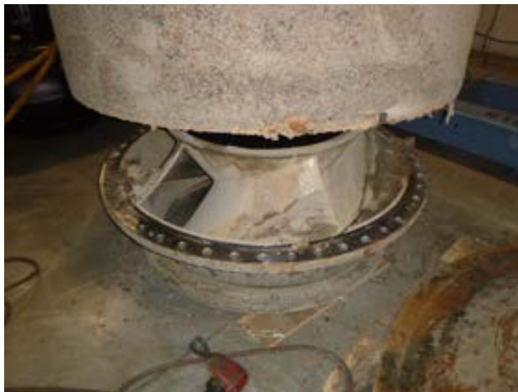
Figure 3-5 ST-5 Impeller with mud deposited on top side of vanes (photo courtesy of KI)
