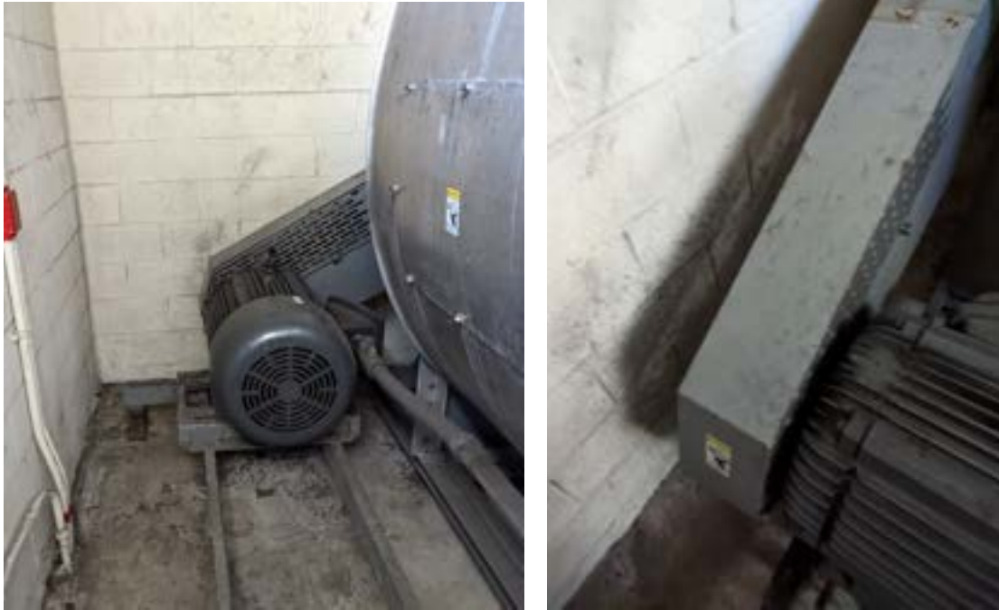
Figure 2-2 Northeast Corner of Supply Fan Room Showing Minimal Maintenance Access for SF-1.
