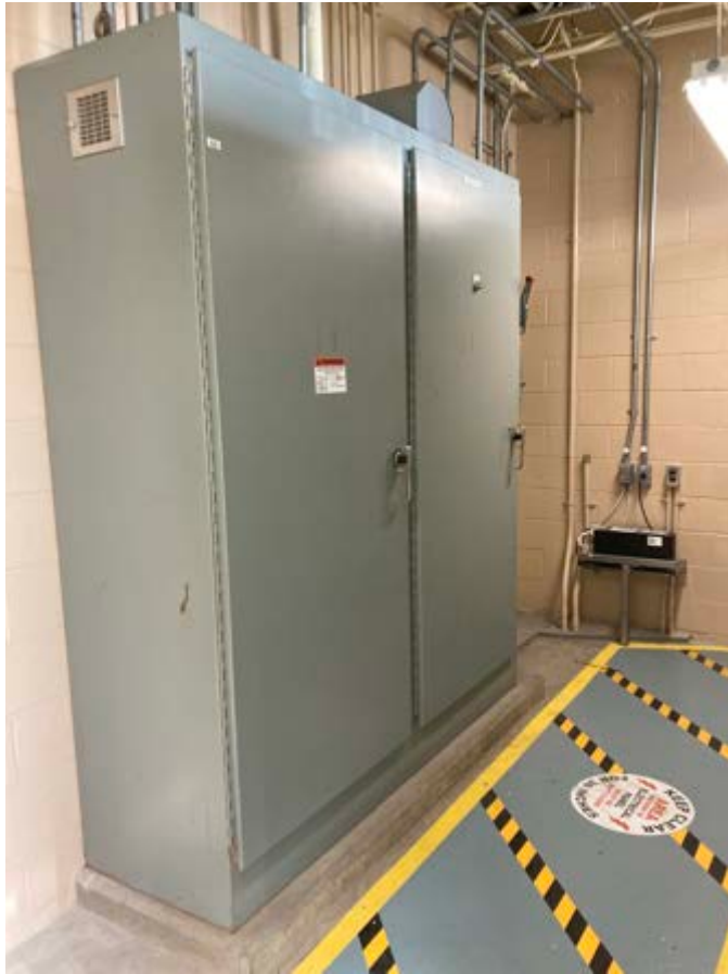
Figure 2-8 Existing Control Panel CP-1A housing Allen-Bradley PLC hardware. CP-1A will be converted to a Marshalling Cabinet under separate CIP.
