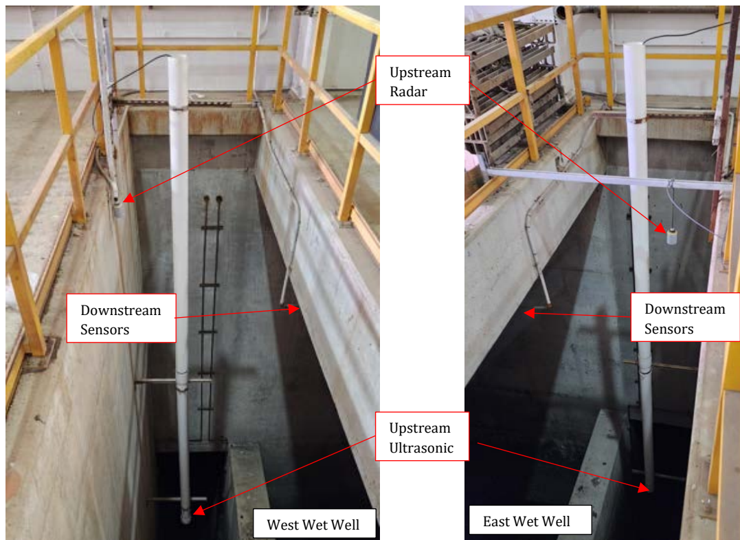
Figure 2-2 Wet Well Level Sensors at Oakwood SPS
