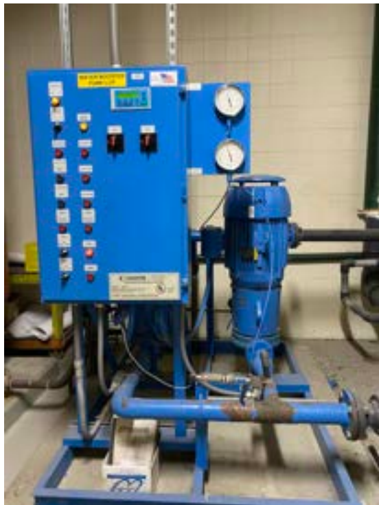
Figure 2-3 Oakwood Screen Facility Booster Pump System
