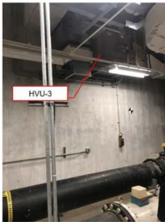
Figure 12-4. HVU-3 Located in Difficult to Access Location Located in Inaccessible Area
