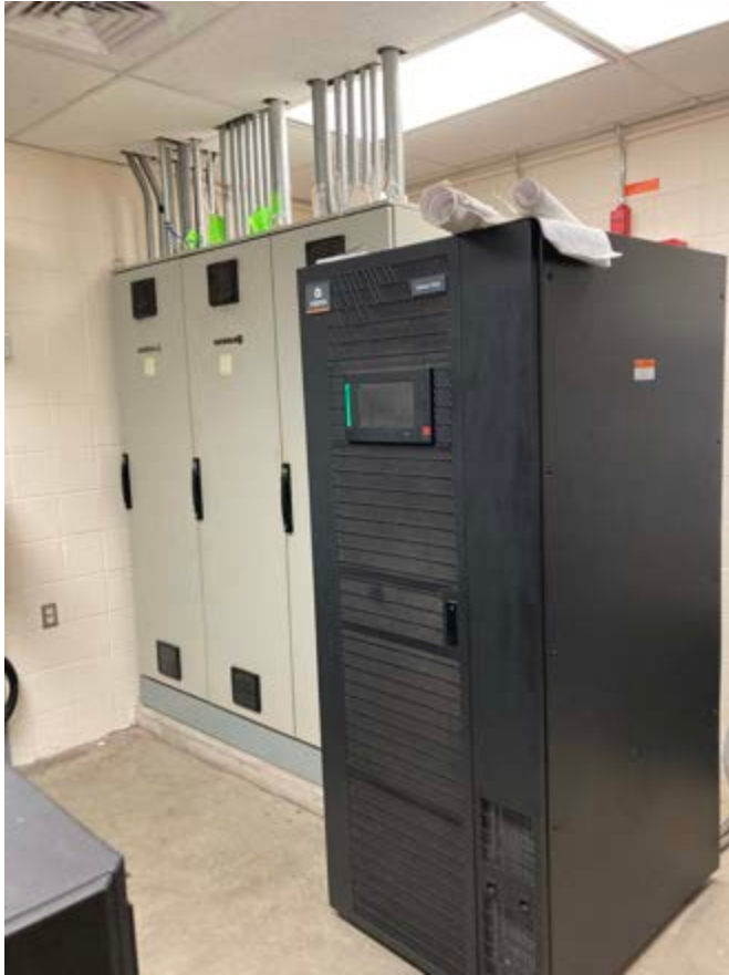
Figure 2-3 Ovation Controller Cabinet, Extended I/O Cabinet, and UPS Cabinet in the Instrumentation and Communication Room
