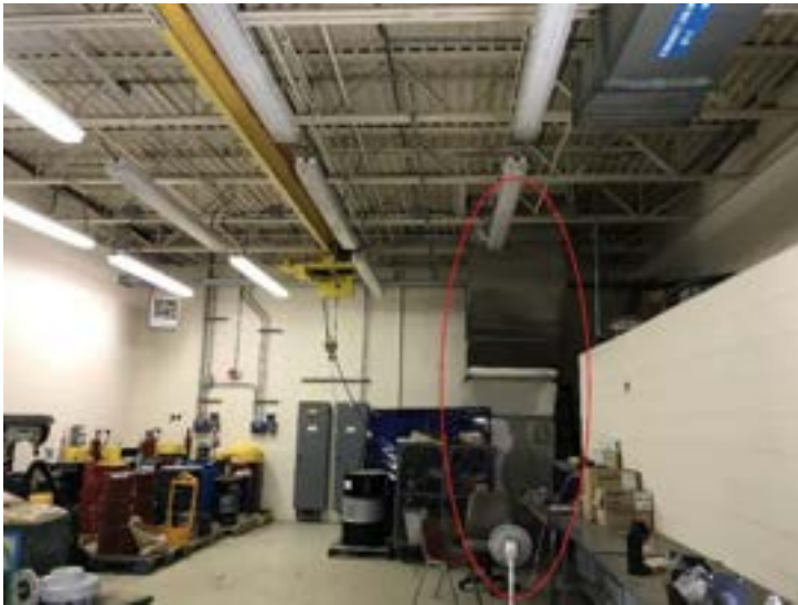
Figure 8-5. Supply Duct for SF-22 Not Enclosed in Fire-Rated Wall
