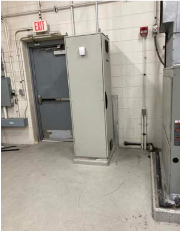
Figure 2-4 Ovation Remote I/O Cabinet in Screening Facility Electrical Room
