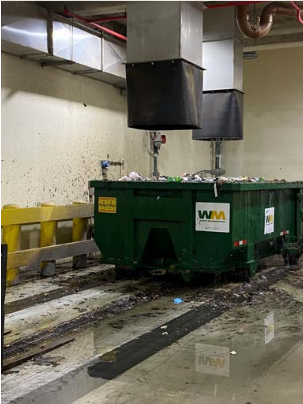
Figure 1.5 – Oakwood CSO RTB Screenings Dumpster Overflowing During Storm Event
