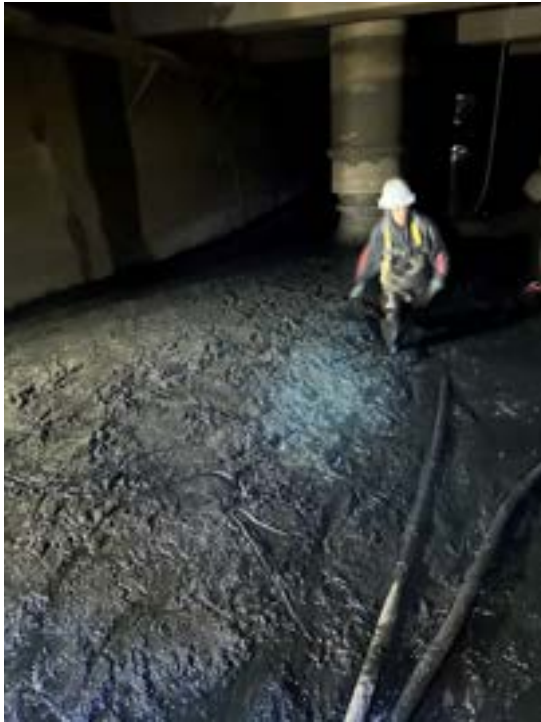
Figure 3-6 Wet Well Debris February 2023, photo courtesy Pullman SST, Inc.
