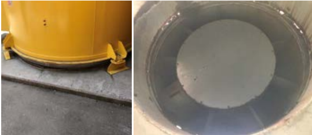
Figure 12-5. Corroded Supply Fan Bases – View from Above (left) and View from Below (right)
