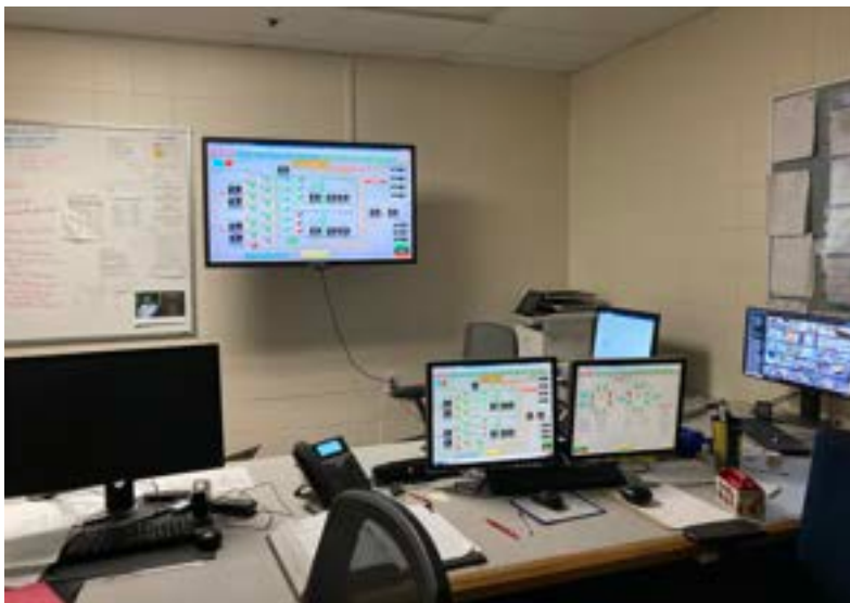
Figure 2-5 Control Room for Oakwood CSO Facility
