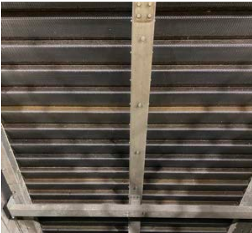
Figure 3-2 Clean Screen #4 after Operation Stopped on 12/15/22
