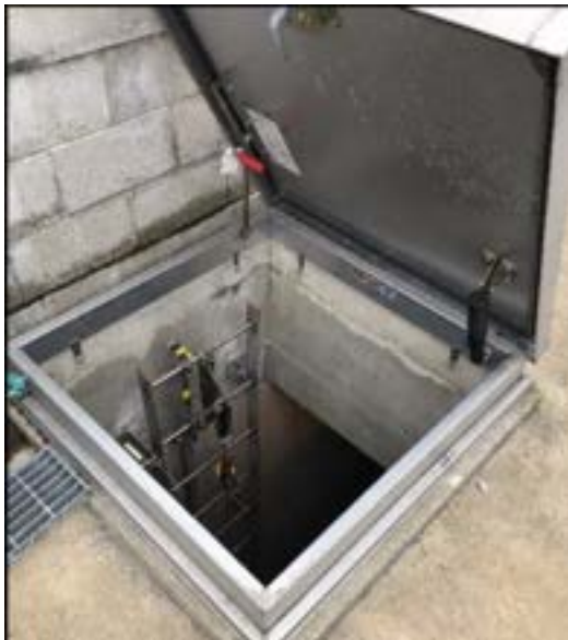
Figure 5-9. Example of Need for Re-orienting the Basin Access Hatches
