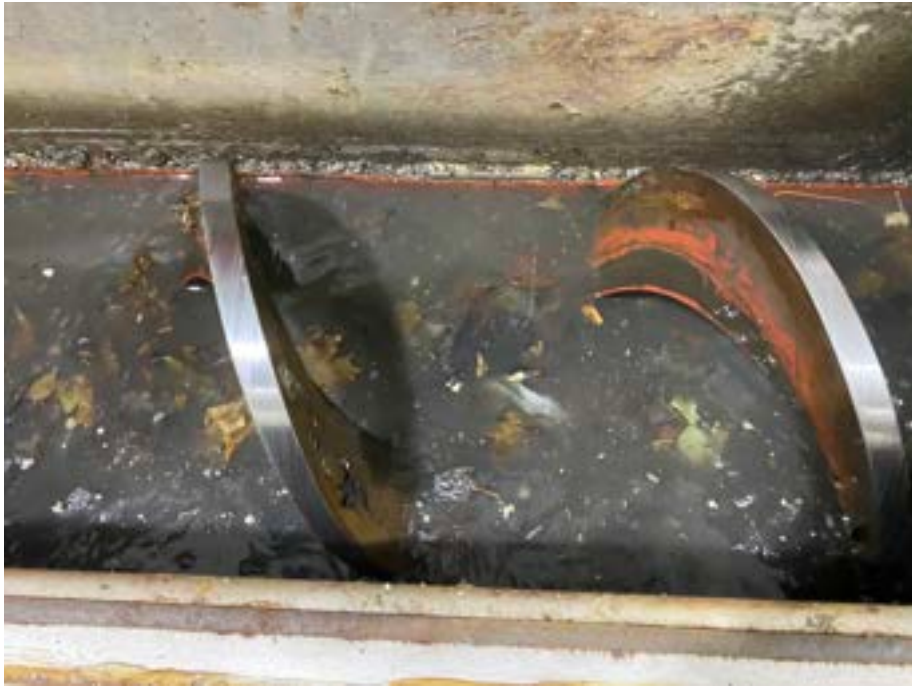
Figure 3-4 Inside operating conveyor between Screens #4 and #6 during wet weather event
