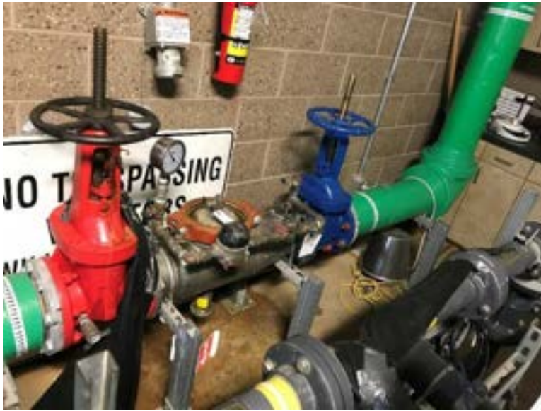
Figure 7-12. Water Spray Near Backflow Preventer
