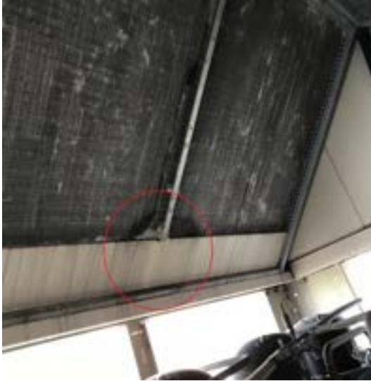
Figure 8-4. Oil on McQuay Unit Condensing Coil
