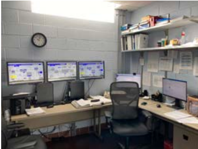
Figure 2-6 Existing Rockwell HMI System in Office
