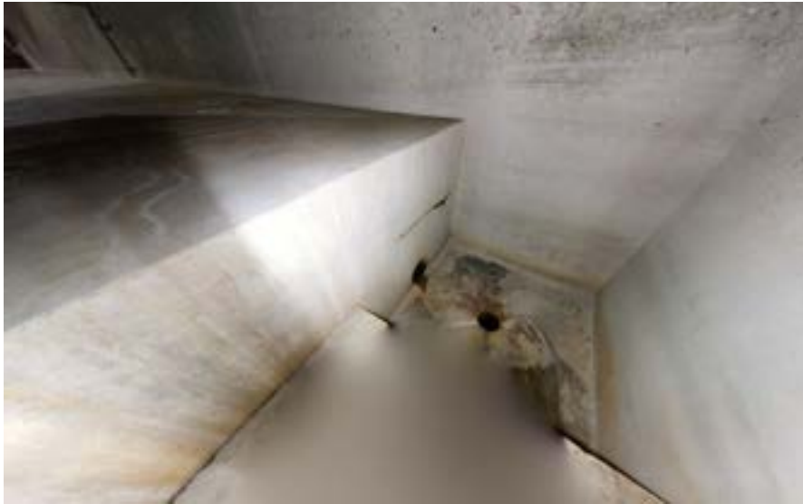
Figure 2-5 Sump at Effluent Side of Oakwood CSO RTB
