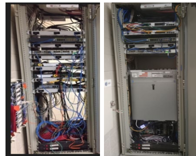
Pre-upgrade and post- within the network cabinet
