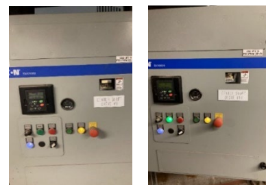
Incinerator nine (Left) Incinerator 10 (Right)
