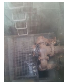
I-Valve Vault at North Service Center
