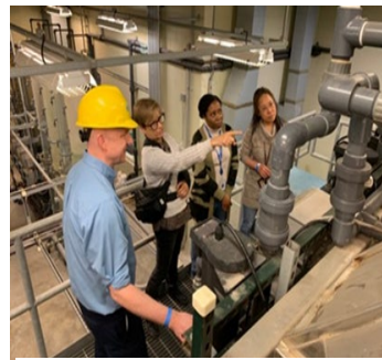
Waterworks Park Pilot Plant
