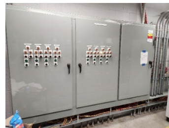
New Baby Creek CSO Screens Control Panel
