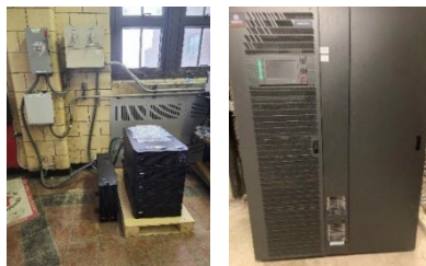
PS1 (left) and PS2 (right) New UPS
