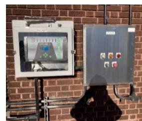
Gas Detection Controller and Alarm Panel
