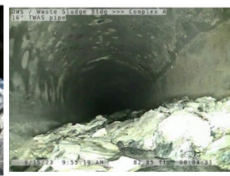
Lining from Pickle Liquor Tank 1
