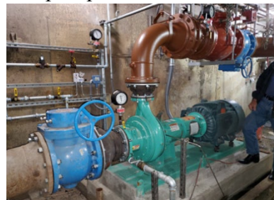
Newly installed SFP No.2
