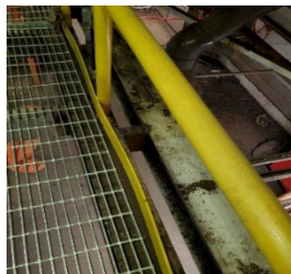
Extra support for maintenance platform
