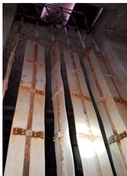
Existing inlet controls
