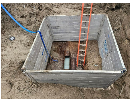
TWAS Line Prepared for Mechanical Cleaning
