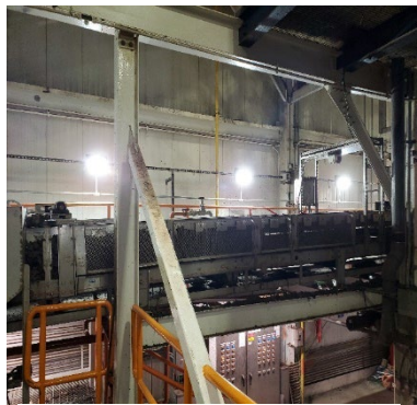
New lights at conveyor K
