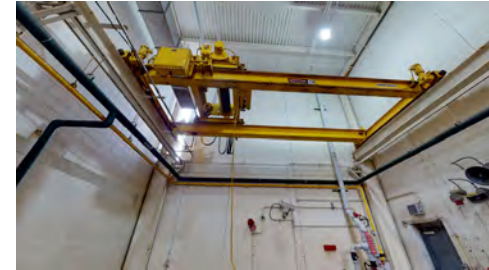
Corroded building crane from failed HVAC system
