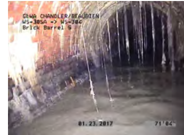
Woodward Sewer System
