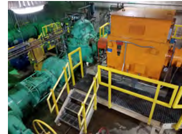
Inside Joy Road Pumping Station
