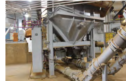
Incineration Complex II, Ash System
