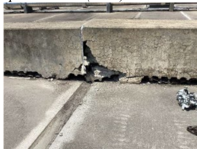
Existing Concrete Enclosure Failure at HS
