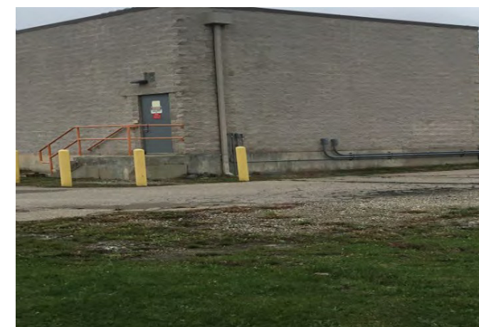
Figure 20. Adams Road Pump Station
