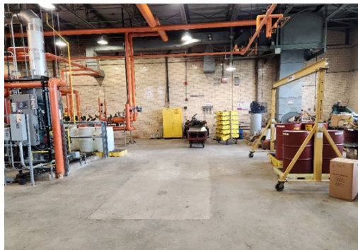
WWP boiler area
