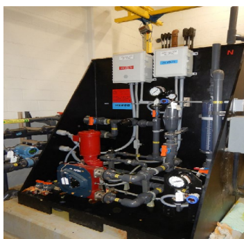
PS-2 Ferric Chloride Pump Skid
