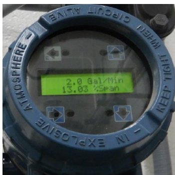
PS-2 Ferric Chloride Flow Meter
