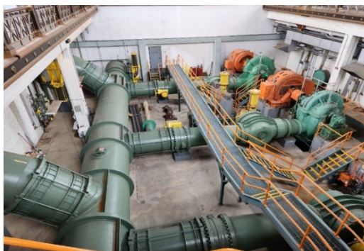
WWP high lift pump area
