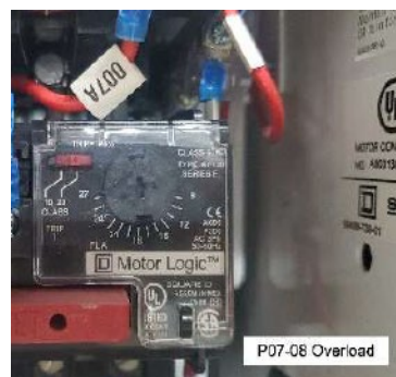
Conveyor P-7/8 Overheated
