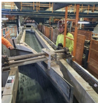
Sludge Bypassing Conveyor P-11/12 Plow
