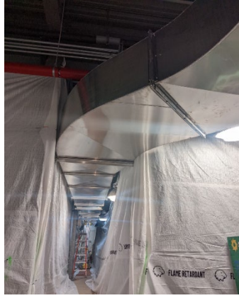
Newly installed ductwork in sedimentation area
