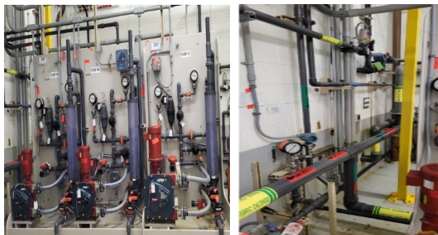
Ferric Pump Room at Pump Station 2
