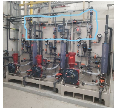
Unreachable Valves at Ferric Chloride Pump Skids
