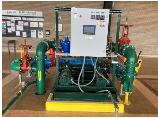
SWWTP raw water screen booster pumps
