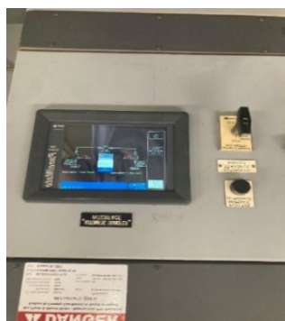
Complex A HMI
