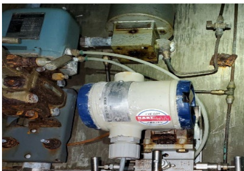
NEWTP old loss of head meter
