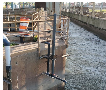
PS-2 Discharge Channel Ferric Chloride Feed
