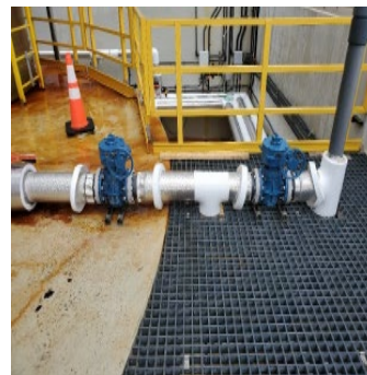
Ferric Chloride Pipe and Valves
