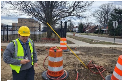
D. Solis checking chlorine residual
