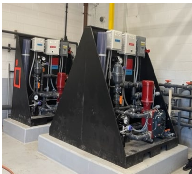
Ferric Chloride Pump Skids
