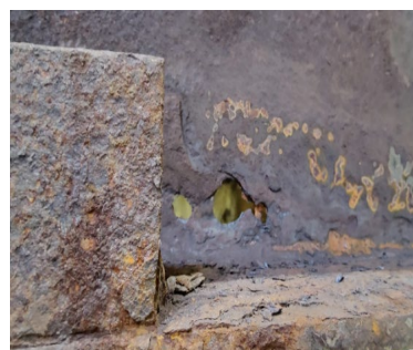
Corroded Framing at PS-1
