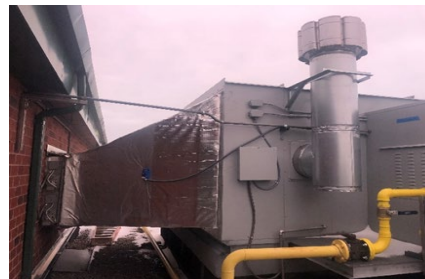
Newly Installed Makeup Air Unit 2 shown above
