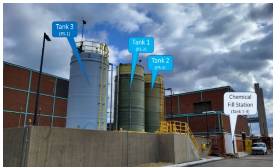
Ferric Storage Tanks at Pump Station 2 (PS2)
