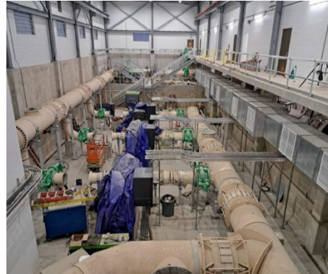
Pump Station 635 Pump Floor
