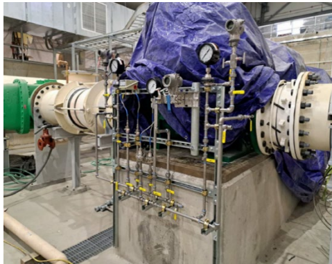
Horizontal Split Case (HSC) pump impulse piping Instrumentation Rack
