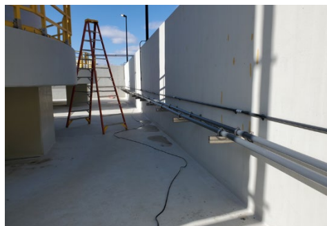
Damaged Ferric Chloride discharge piping is replaced by the Contractor shown above
