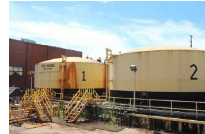
Ferric Chloride Storage and Containment Area
