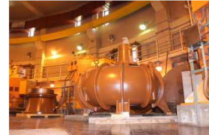
Main Raw Sewage Pumps at Pump Station 2
