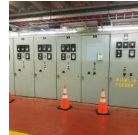
Representative Switchgear to be Replaced under CIP 111001
