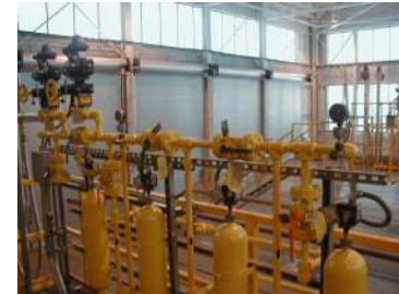
Chlorination Building, Inside
