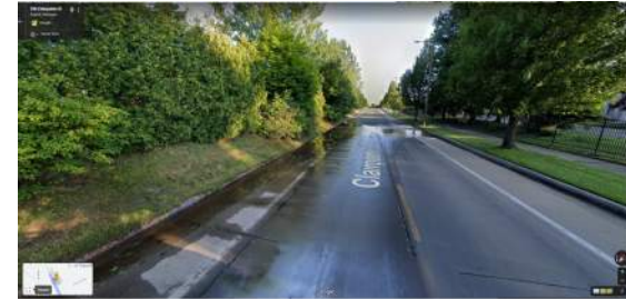
Photo of the berm leaking into Clairpointe
