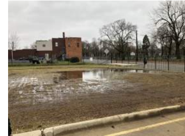
Poor Drainage at Leib
