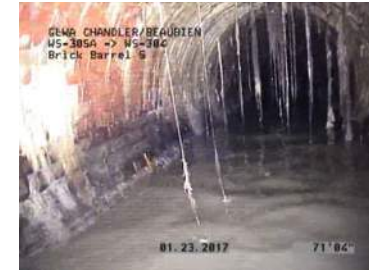
Woodward Sewer System
