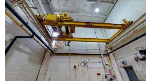
Corroded building crane from failed HVAC system
