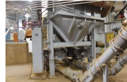
Incineration Complex II, Ash System
