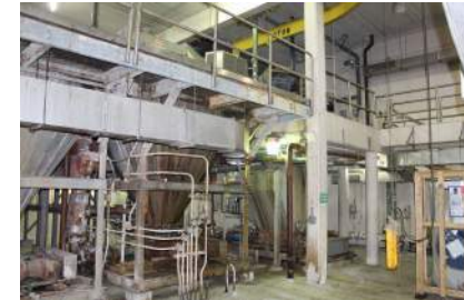
Primary Circular Scum House, Inside
