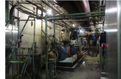
Sludge Feed pump in Complex A
