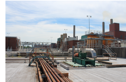
Aeration Basin 1 and ILP's 1 and 2
