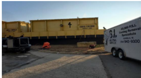
Ferric Tanks Rubber Lining
