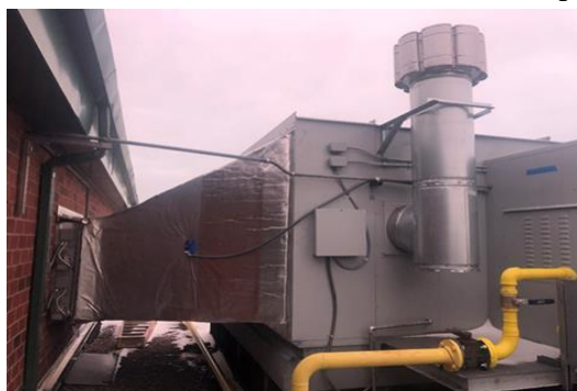
Newly Installed Makeup Air Unit No. 2
