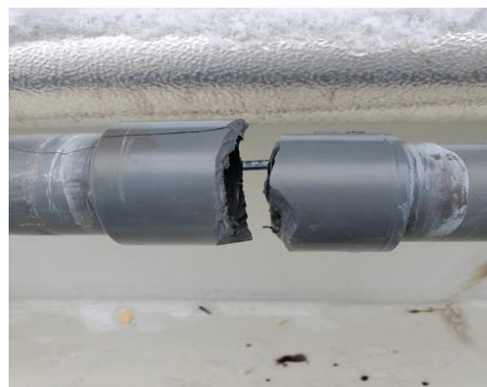
Damage to ferric chloride discharge piping
