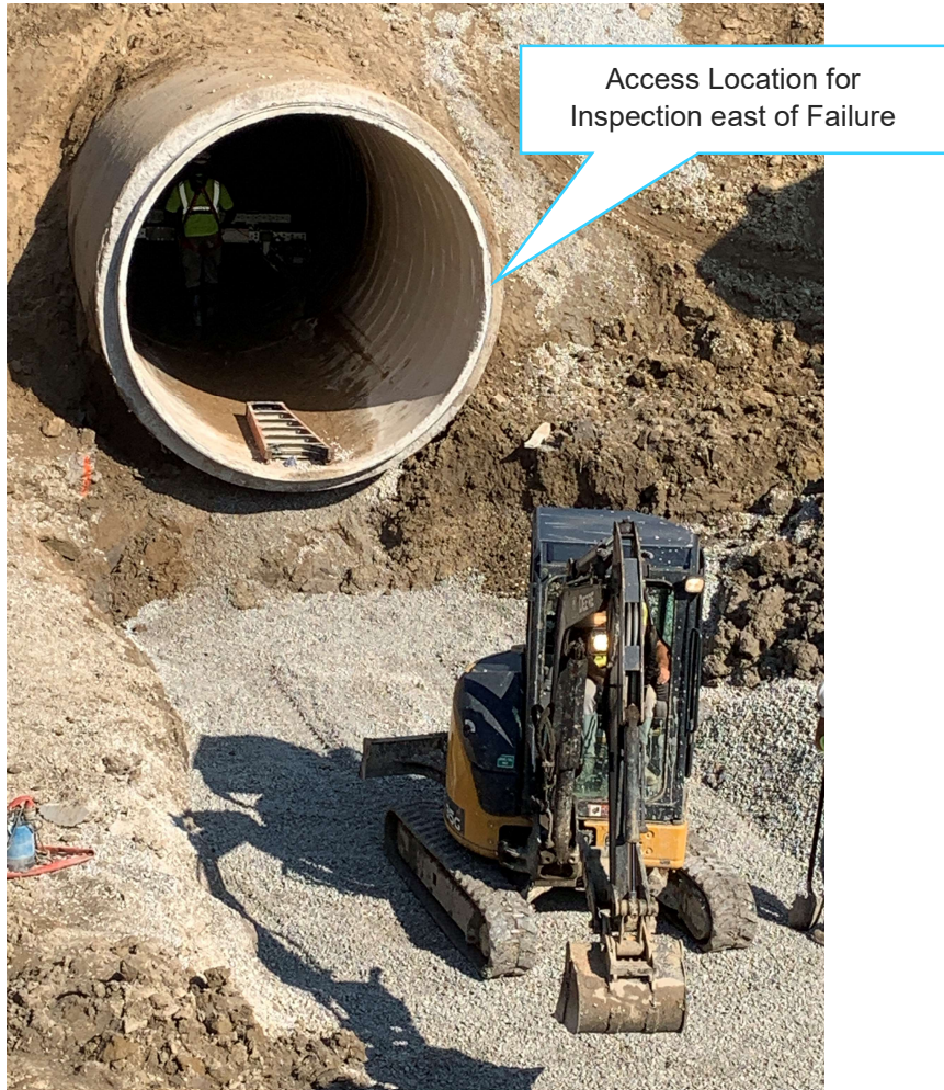
Figure 1.2: Access for the Inspection was the Failure Location
