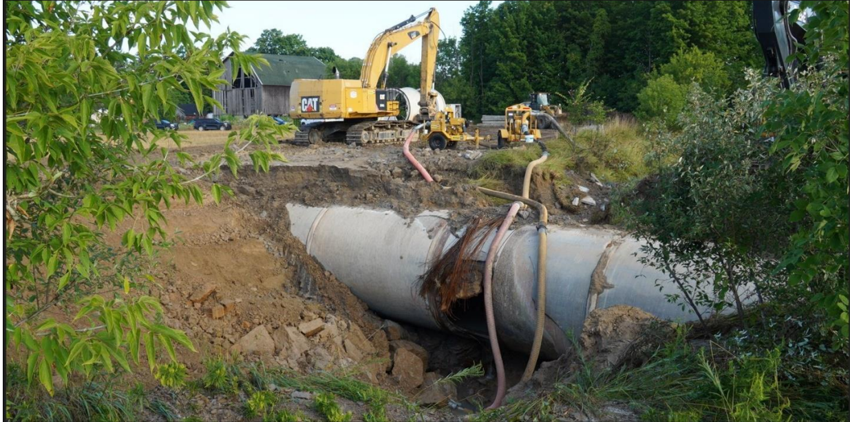
Figure 3. GLWA experienced a significant water main failure on its 120-inch Transmission Main originating from the Lake Huron Water Treatment Facility on August 13 th , 2022, at 4:30 AM (image obtained from GLWA's social media post).
