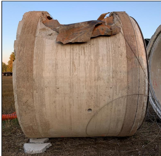
Figure 4a. Side profile image of the ruptured pipe. Note that the rupture occurred near the invert and on the south side of the pipe.
