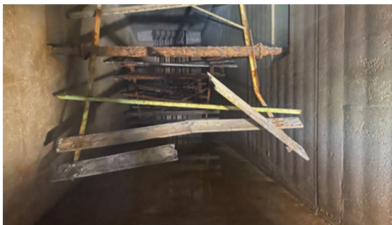
Existing flocculator equipment Sedimentation Basin #1
