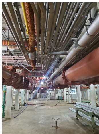
Corroded pipe before replacement
