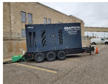
Emergency generator/Low Lift area
