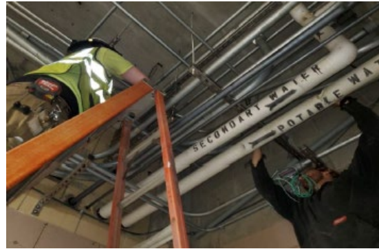
Conduits in Chemical Building
