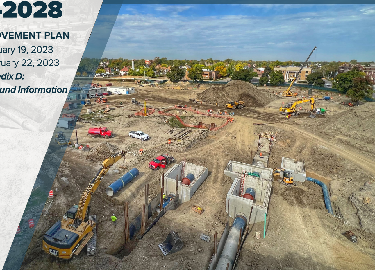
Water Works Park Water Treatment Plant Yard Piping, Valves, and Venturi Meters Replacement Photo submitted by: Jacob Magnum of Water and Field Services
