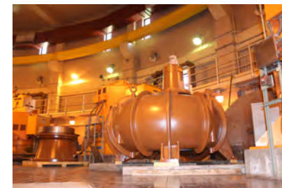
Main Raw Sewage Pumps at Pump Station 2
