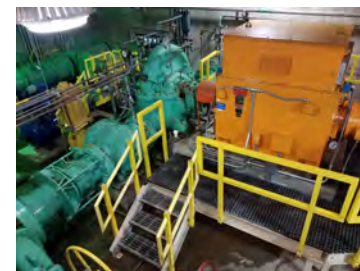
Inside Joy Road Pumping Station
