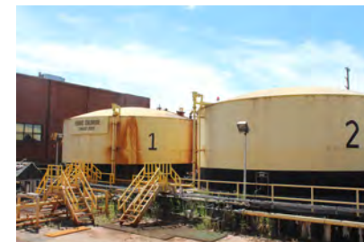
Ferric Chloride Storage and Containment Area
