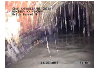
Woodward Sewer System
