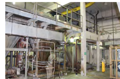
Primary Circular Scum House, Inside
