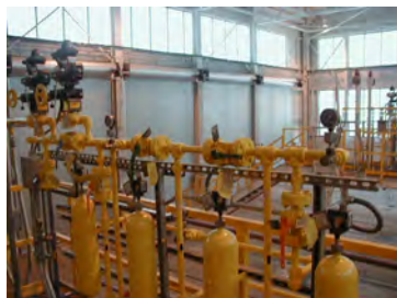
Chlorination Building, Inside
