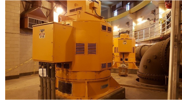
Main Raw Sewage Pumps at Pump Station 2
