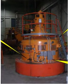
Pump at the Northeast Pumping Station
