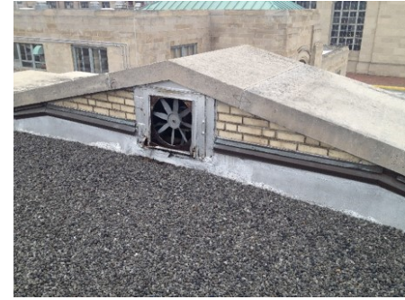
Roof in need of repair
