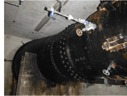
Water production flow metering device
