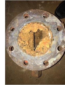
The photo shows the condition of the heating system hot water piping.
