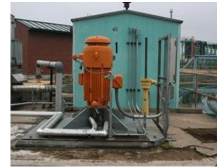
Return activated sludge pump and Motor Control Center building
