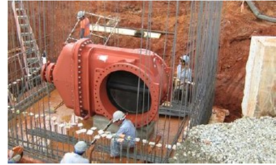
A large valve for a transmission pipe
