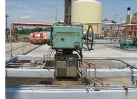
Equipment for aeration system
