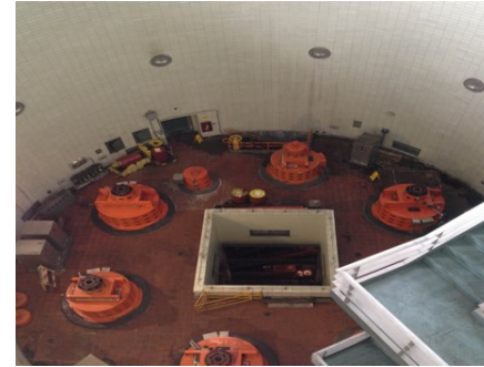
Low Lift Pumping Plant at Northeast WTP
