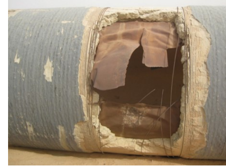
Example of a failed water main
