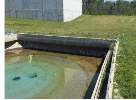
Raw sludge clarifier at Lake Huron WTP
