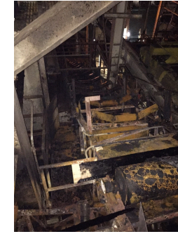
Picture from left to right Sludge Conveyer G Damaged by Fire and Conveyer B in the Complex – II Dewatering Building and Fire Damaged Conveyer H in Complex-II Incinerators Building
