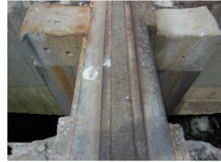
Piece of movable dam at DRO-2
