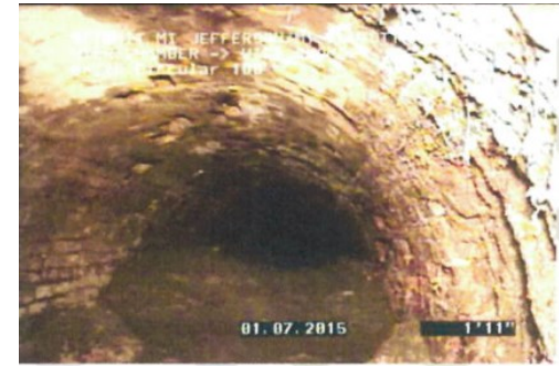
Sewer tap piping in B009 outfall (left) and sludge buildup and poor masonry in B007 outfall (right)
