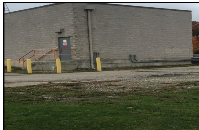
Figure VI-20. Adams Road Pump Station
