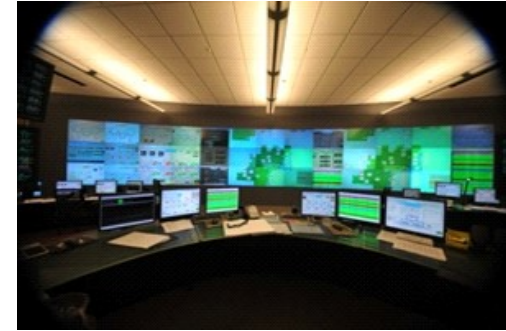
A system control room
