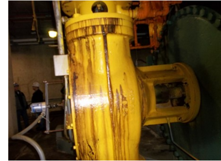
Oil hydraulic valve actuators leaking oil
