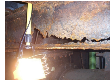
Deteriorated support beams holding up Low Lift Station. Dewatering and Sump Pumps at Elev. 42'-0" (left). Deteriorated grating and access ship's ladder in Low Lift Station - Looking down at Elev. 50'-0" and 42'-0" from Elev. 62'-0" (right).
