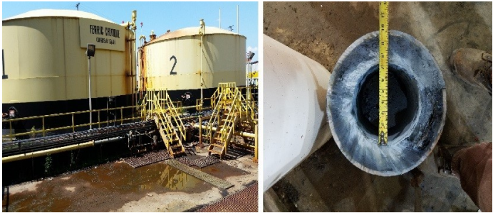
Ferric Chloride Tanks at Pump Station 1
