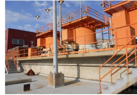
Intermediate Lift Pump Station N.2
