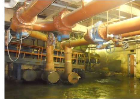
Sludge Feed Pumps
