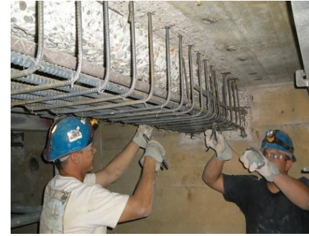
Lake Huron WTP Electrical Tunnel
