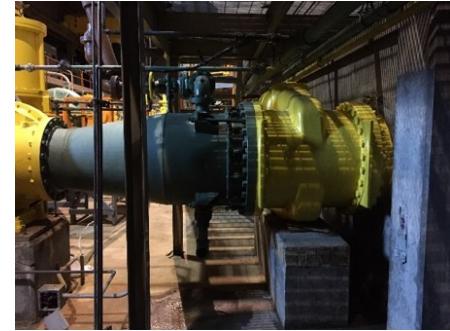
Isolation gate valves
