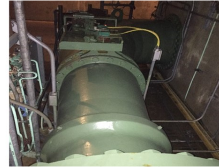
Raw Water Flow Meter
