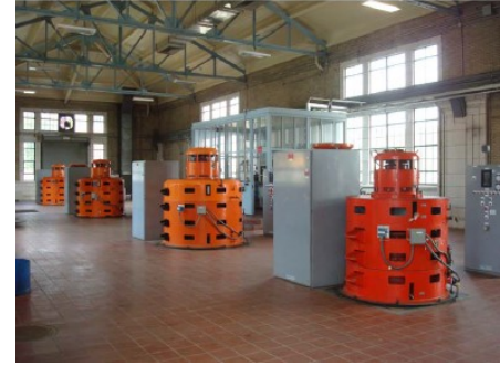
Sanitary pumps at Fairview Pumping Station
