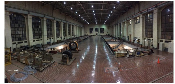
High Lift Station viewed from Low Lift Station operating floor showing high lift pump pits and windows to be replaced.
