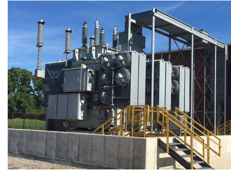
The new 3rd 120/13.8 kV Transformer installed and owned by the Great Lakes Water Authority waiting for the 3rd Primary Electric Feed Line to be installed and energized
