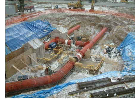
Example of a large pipe and valve installation
