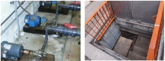
Retrofitted chemical feed pump replacement at Puritan-Fenkell RTB and makeshift wooden stairs to enter Basin Valve Gallery
