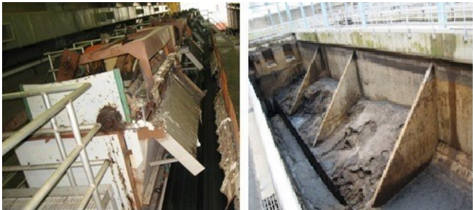
WRRF Pumping Station 2: Bar Racks and Grit Collection System
