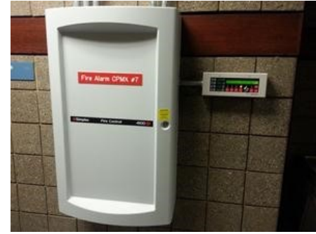
Fire alarm system
