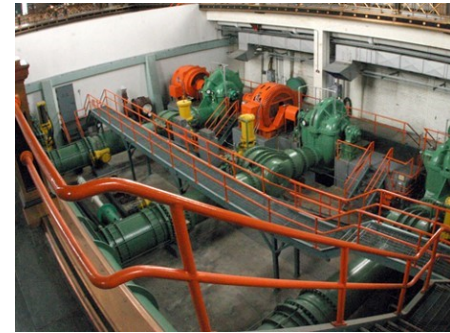
Pumps and Piping
