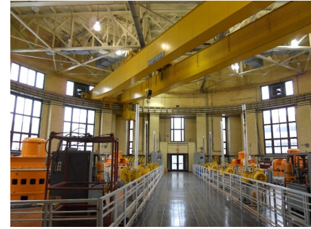
Pump Station 1 Interior
