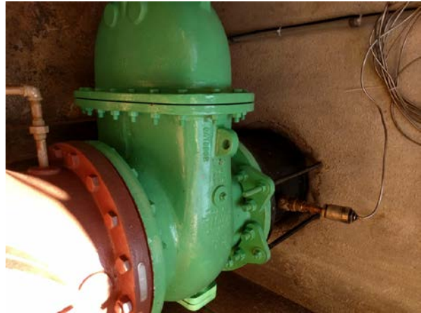
Chene and Maple PRV New gate valve installation at the site to allow for more reliable shutdown capability at the site.
