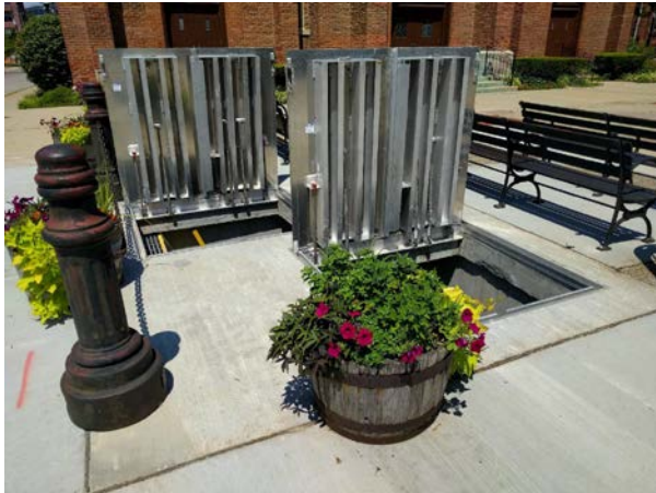
Porter and 6th PRV At grade access hatches were incorporated into the outdoor seating area of the Most Holy Trinity Church at the site. Careful coordination took place to make sure that the Church's outdoor seating area was not disrupted with the final layout of the hatches.
