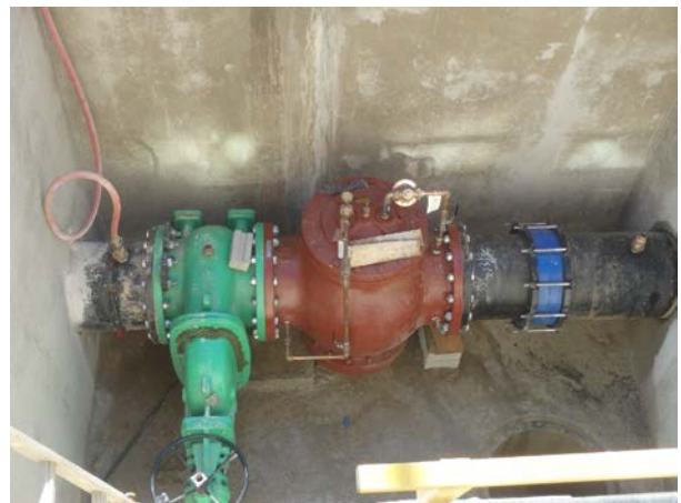
Park and Elizabeth PRV Final piping layout of completed PRV replacement. PRVs were replaced in full with all new pilot systems resulting in improved reliability. In addition, a new gate valve isolation was provided at the site such that the PRV could be taken out of service for maintenance in the future with less impacts to customers in the vicinity of the site.
