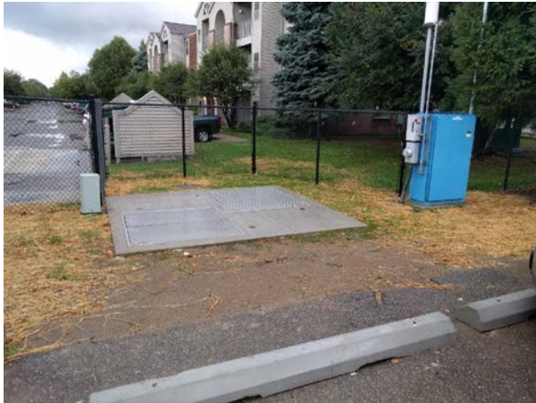
Chene and Maple PRV Final restoration at Chene and Maple site. Double hatch access allows for improved safety and ease of access.
