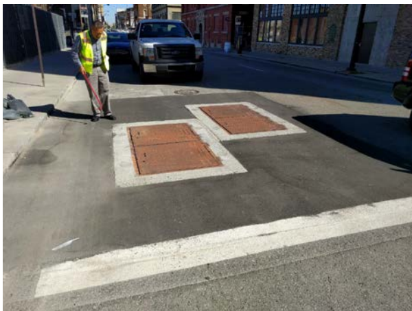
Park and Elizabeth PRV Final restoration photo showing double hatch access to the upgraded vault. Double hatch will facilitate operations and maintenance activities at the site.
