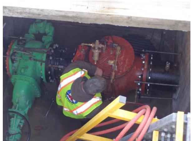
Porter and 6th PRV Final piping layout of completed PRV replacement. PRVs were replaced in full with all new pilot systems resulting in improved reliability. The vault expansion at the site allows for more room for maintenance activities within the vault.
