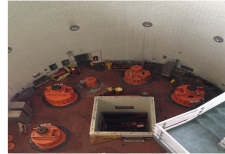
Low Lift Pumping Plant at Northeast WTP
