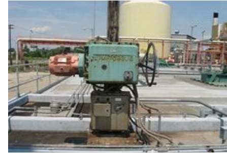
Equipment for aeration system
