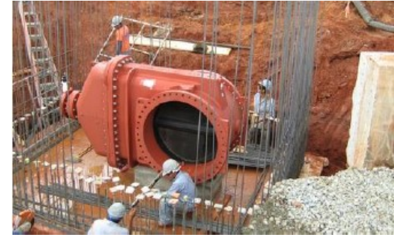
A large valve for a transmission pipe
