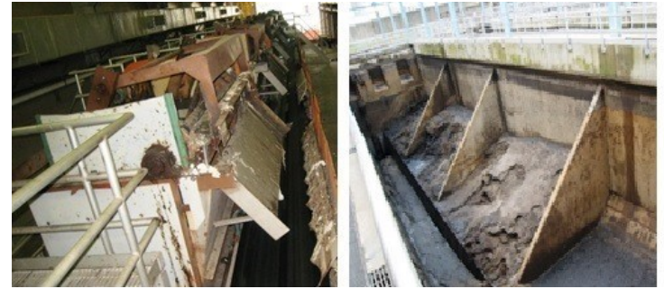
WRRF Pumping Station 2: Bar Racks and Grit Collection System
