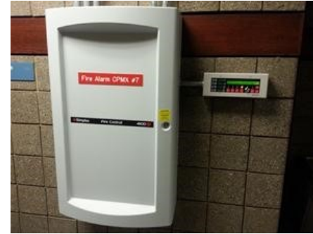
Fire alarm system
