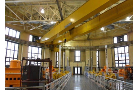
Pump Station 1 Interior
