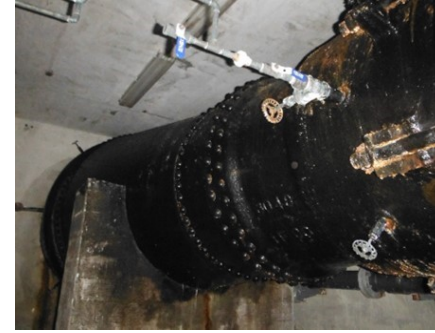
Water production flow metering device
