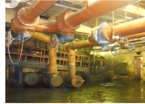
Sludge Feed Pumps
