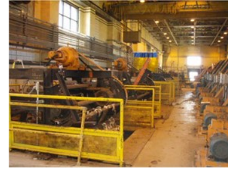
Rack and Grit
