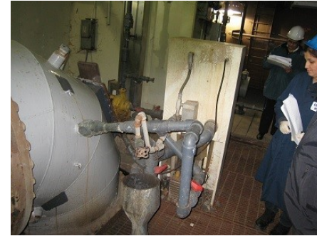
The RAS-3 sampling station in the basement of Intermediate Lift Pump No. 2 (ILP No. 2) Building samples the return activated sludge flows to Aeration Deck No.4
