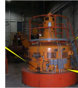
Pump at the Northeast Pumping Station
