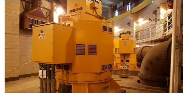
Main Raw Sewage Pumps at Pump Station 2
