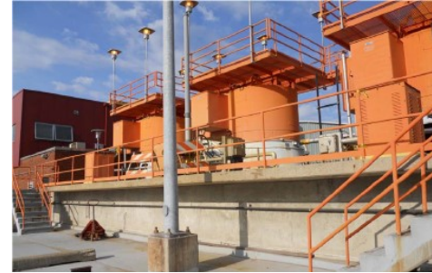
Intermediate Lift Pump Station N.2
