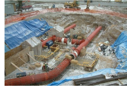
Example of a large pipe and valve installation
