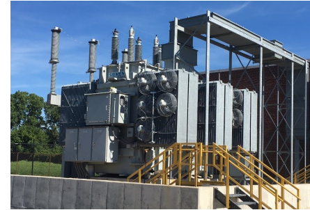
The new 3rd 120/13.8 kV Transformer installed and owned by the Great Lakes Water Authority waiting for the 3rd Primary Electric Feed Line to be installed and energized
