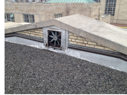
Roof in need of repair
