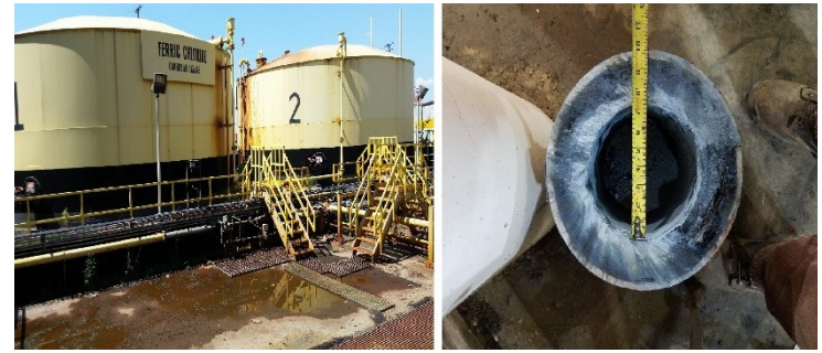
Ferric Chloride Tanks at Pump Station 1
