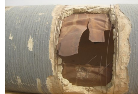
Example of a failed water main
