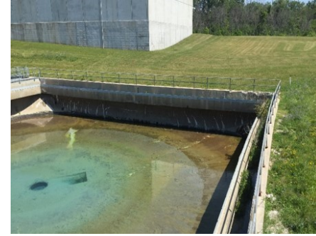
Raw sludge clarifier at Lake Huron WTP
