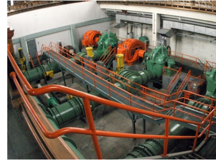
Pumps and Piping
