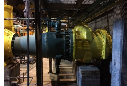
Isolation gate valves
