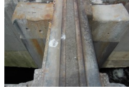
Piece of movable dam at DRO-2
