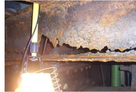
Deteriorated support beams holding up Low Lift Station. Dewatering and Sump Pumps at Elev. 42'-0" (left). Deteriorated grating and access ship's ladder in Low Lift Station - Looking down at Elev. 50'-0" and 42'-0" from Elev. 62'-0" (right).
