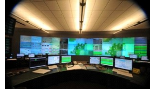
A system control room
