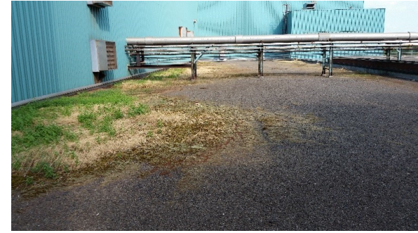
Photo of Complex – I Dewatering Roof at the WRRF. Complex – II Incinerator ($1.8M) and Complex – II Dewatering ($1.0 M) replacement are under consideration to be part of fire remediation project
