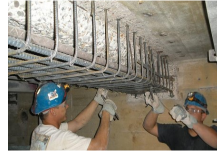
Lake Huron WTP Electrical Tunnel
