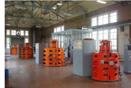
Sanitary pumps at Fairview Pumping Station
