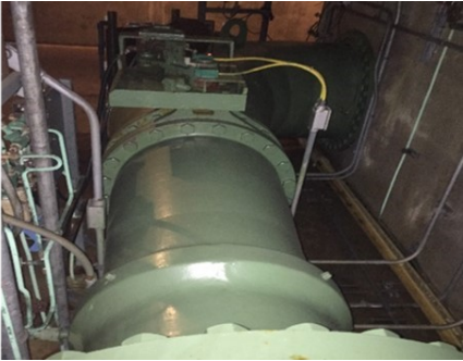
Raw Water Flow Meter
