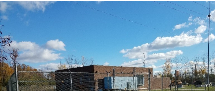
Ypsilanti Pump Station
