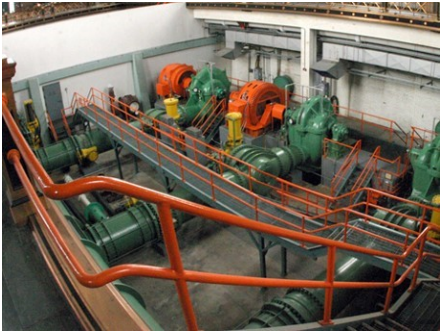
Pumps and Piping
