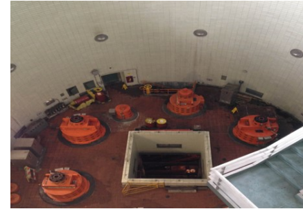
Low Lift Pumping Plant at Northeast WTP
