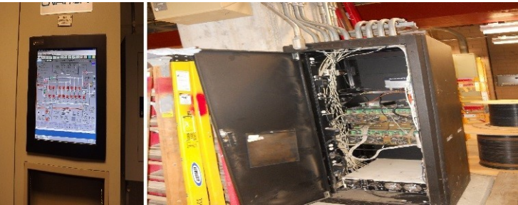
Ovation hardware and screens
