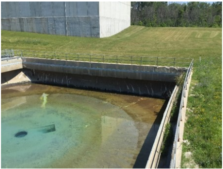
Raw sludge clarifier at Lake Huron WTP
