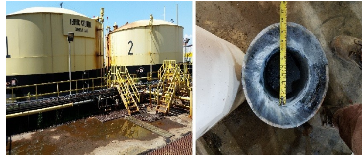
Ferric Chloride Tanks at Pump Station 1
