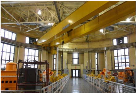
Pump Station 1 Interior
