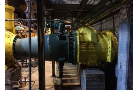
Isolation gate valves
