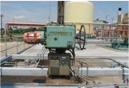
Equipment for aeration system
