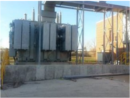
Electrical Duct Bank
